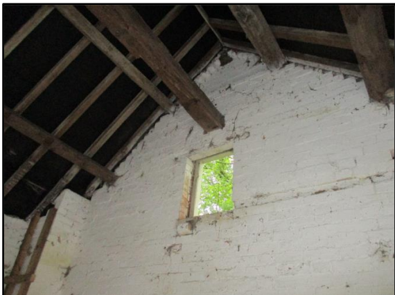
Plate 11: showing opening within the southern gable of B2 through which brown long-eared bats are entering the building.
