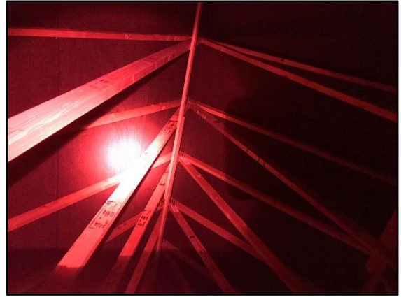
Plate 8: showing a typical view of the roof structure of the garage (B3).
