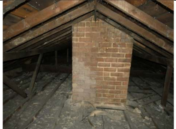
Photograph 20. The enclosed roof void within the main part of the house (north section)
