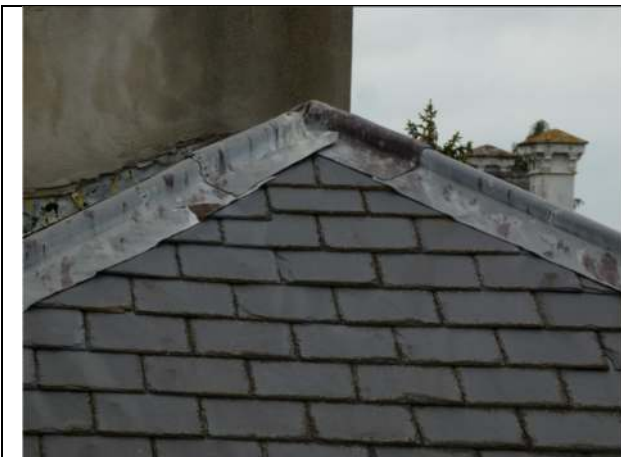
Photograph 9. Example of the slates on an east-facing roof pitch of the house
