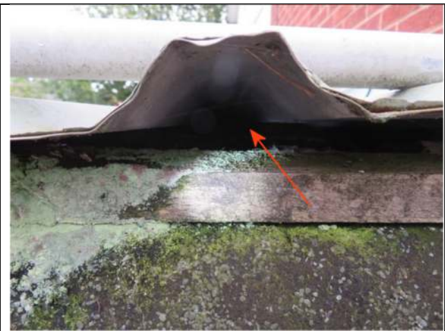
Photograph 16. Example of a gap under the roof of the single-storey section at the eastern end of the house
