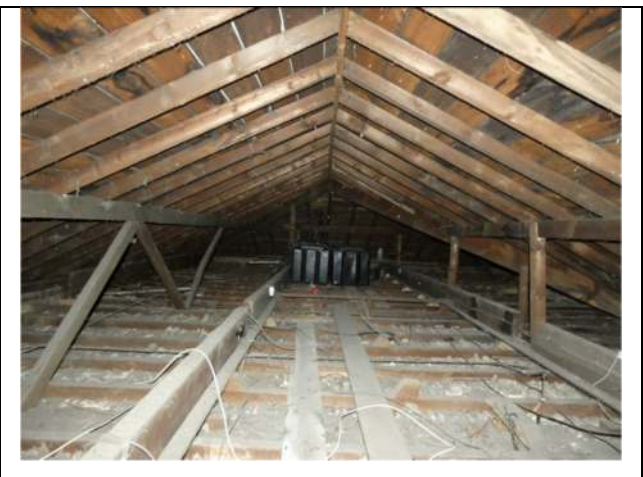
Photograph 18. The enclosed roof void within the main part of the house (west section)
