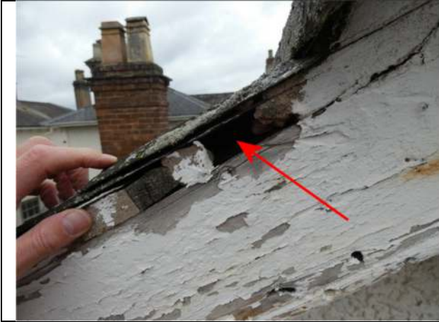
Photograph 13. Opening under a slate above the half gable on the central part of the house
