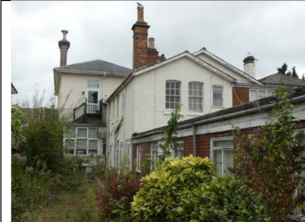
Photograph 7. The south elevation of the central and eastern sections of the house
