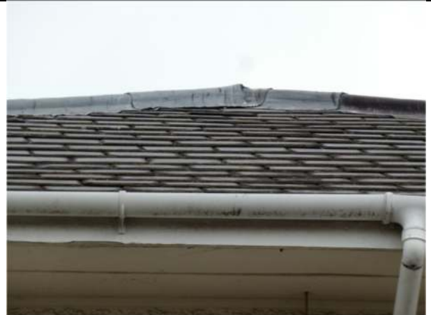
Photograph 8. Example of the slates on the west-facing roof pitch of the house
