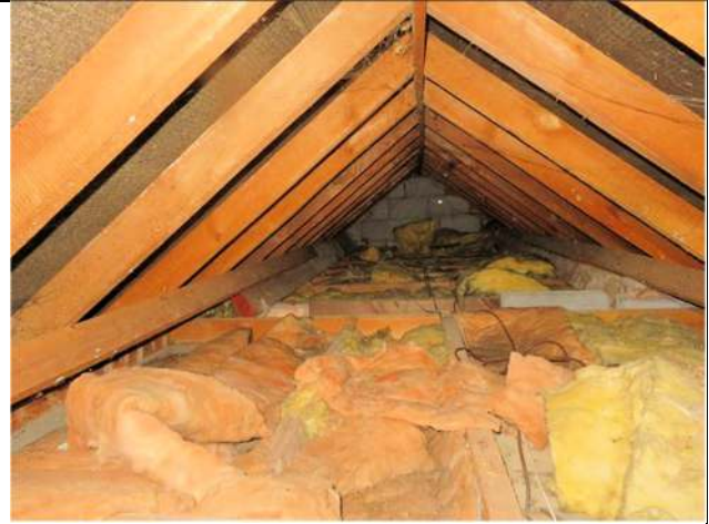
Photograph 32. The section of enclosed roof void within the gabled projection to the south on the cottage
