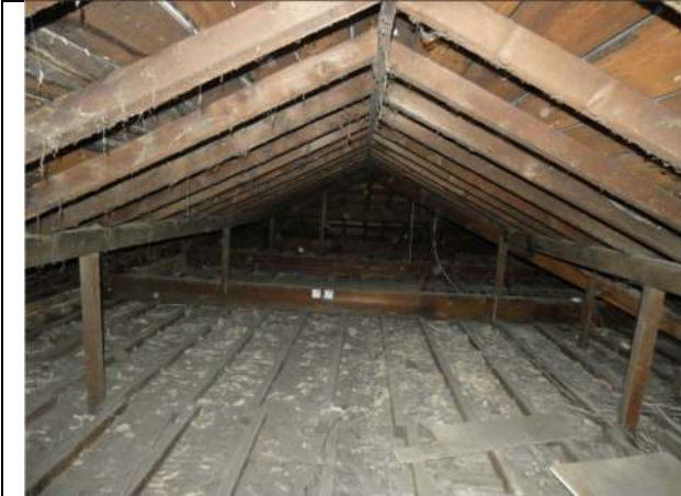
Photograph 19. The enclosed roof void within the main part of the house (south section)
