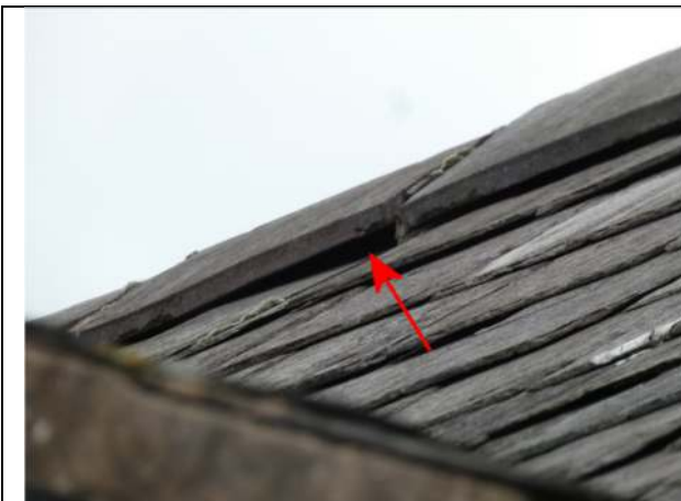
Photograph 27. Opening under a ridge tile on the cottage
