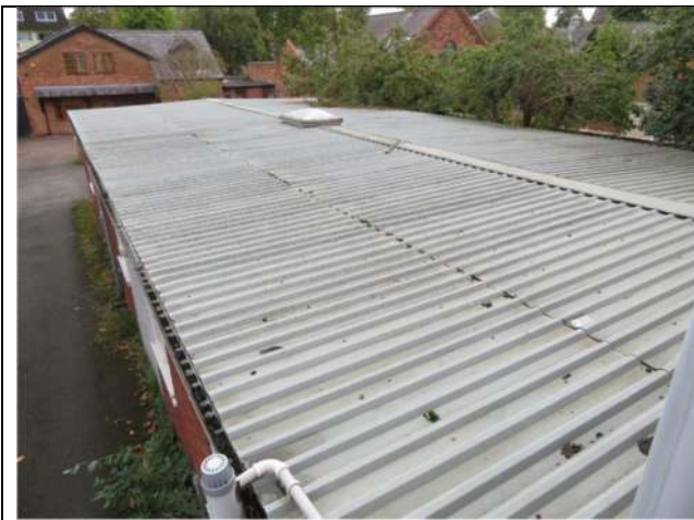
Photograph 15. The roof of the single-storey section at the eastern end of the house
