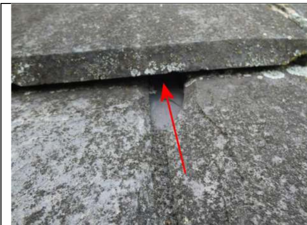
Photograph 11. Opening under a ridge tile on the central part of the house
