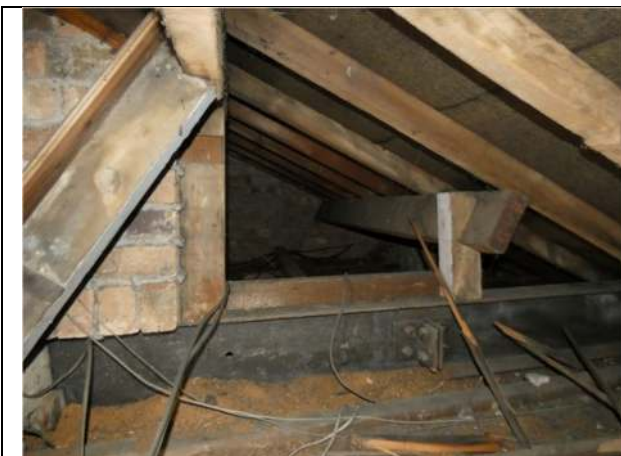
Photograph 23. The enclosed roof void in the central part of the house (to half gable)
