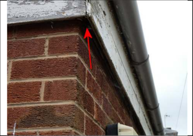
Photograph 14. Gap under the soffit at the north-east corner of the main part of the house
