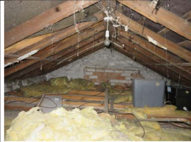
Photograph 31. The section of enclosed roof void within the main part of the cottage
