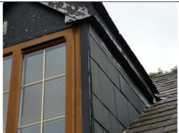
Photograph 28. Example of sealed hanging slates on the dormer window on the western side of the cottage
