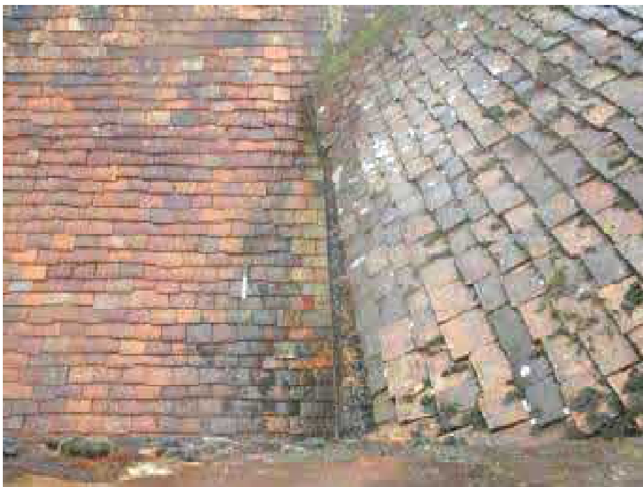
Blocked and leaking gutters
