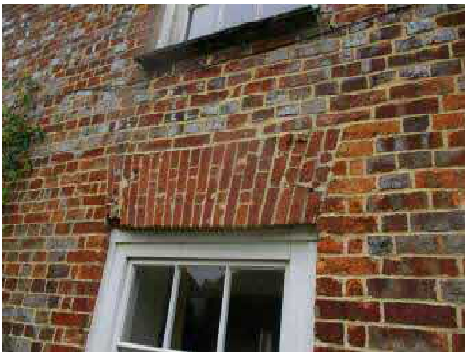
Lintel dropped right hand side
