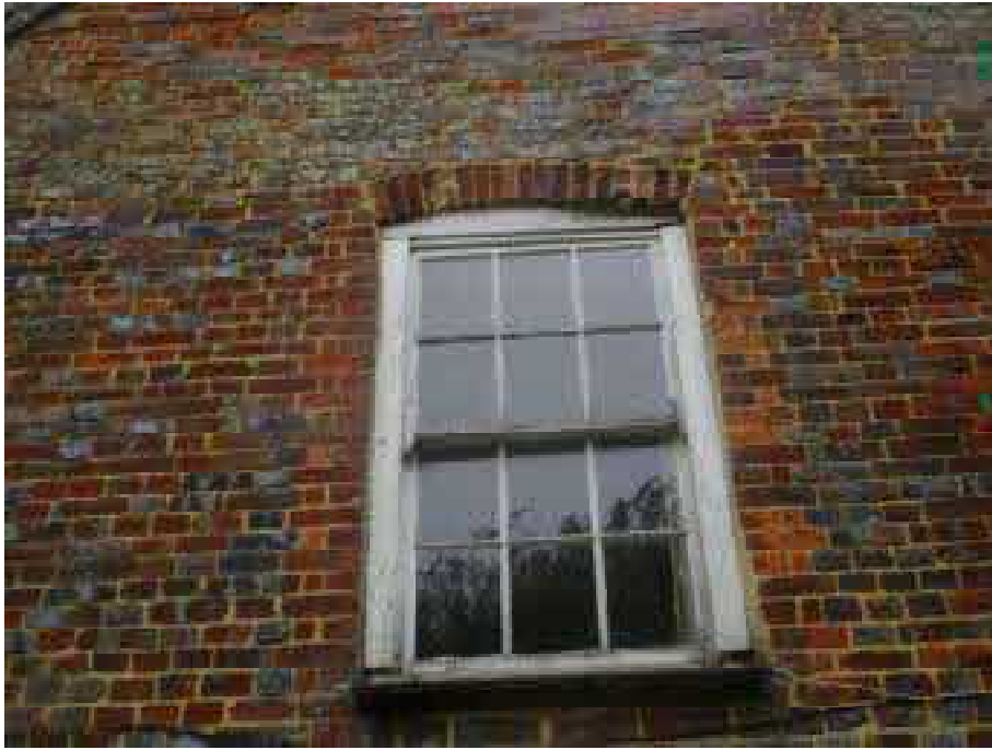
Decay in windows
