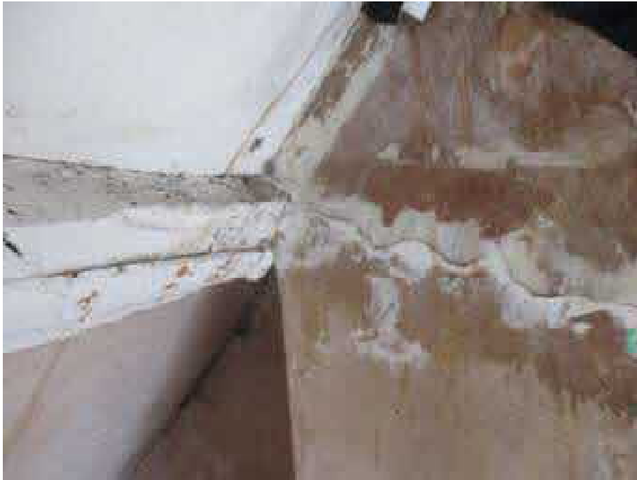
Decay in purlin built into chimney
