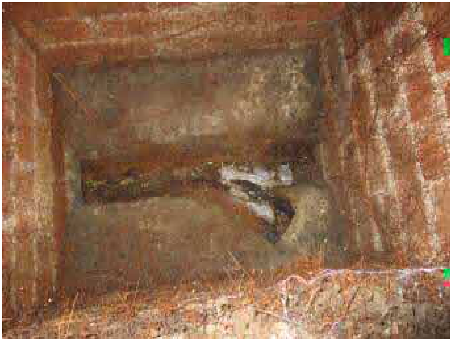
Roots in drain
