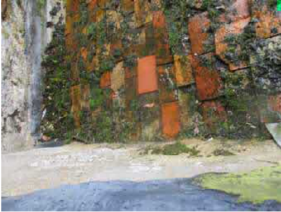
Frost damage and moss to rear valley
