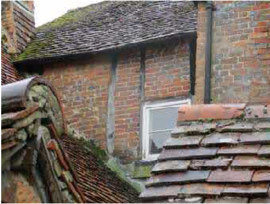
Gutters splashing back to walls
