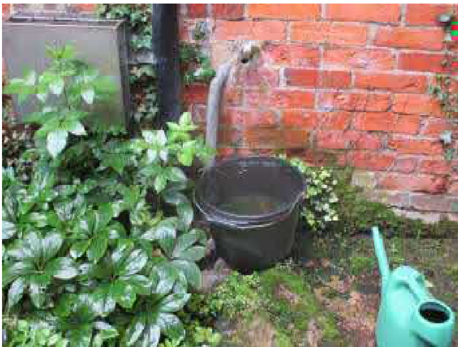
Leaking overflow from toilet
