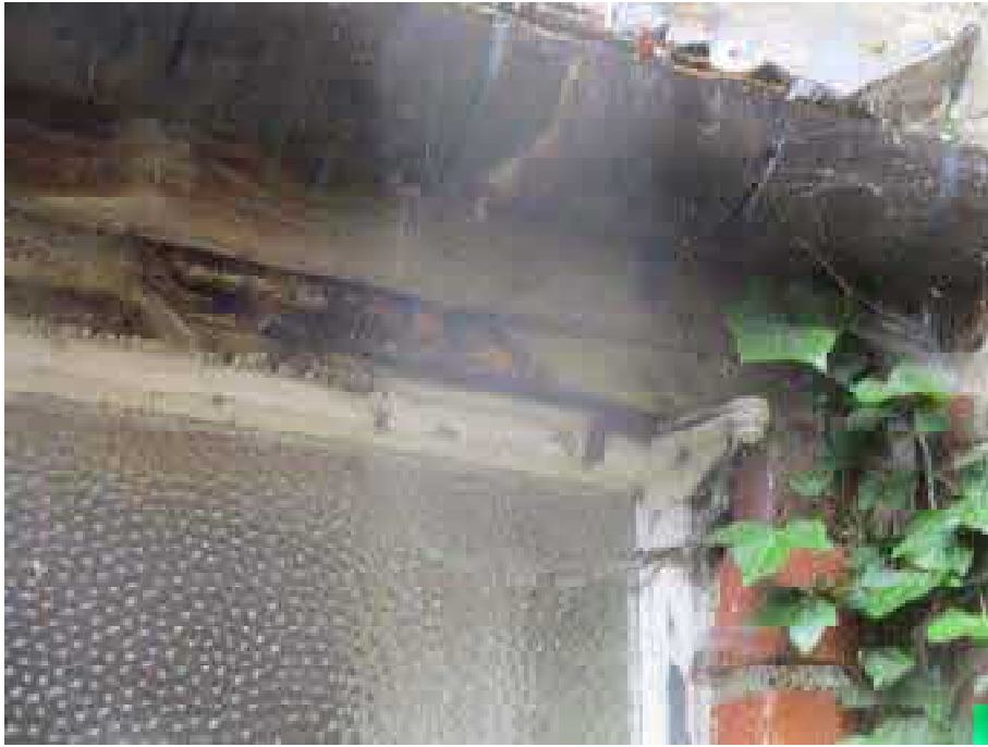
Rotting lintel over WC window
