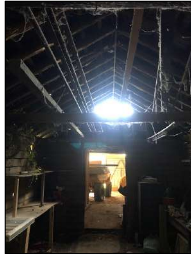
Photograph 6: The internal aspects of building B1B. Photograph taken looking east with building B1A in the background.
