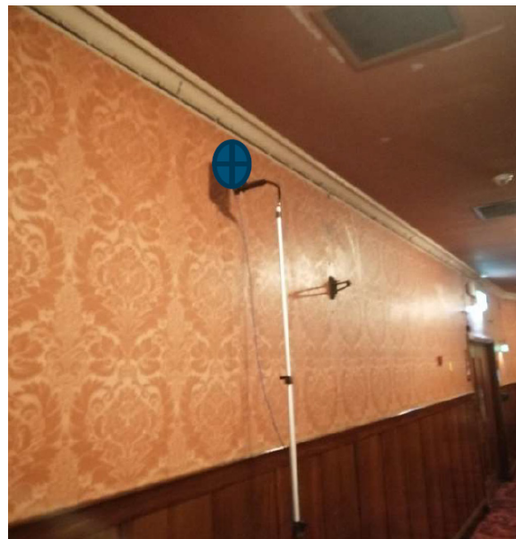
Location AP A11 - Stalls level - unit installed at high level close to existing cabling
