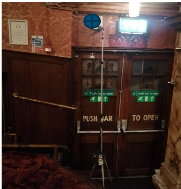
Location AP A6 - Stalls level - unit to be fixed above door in close proximity to existing wall mounted services and cabling
