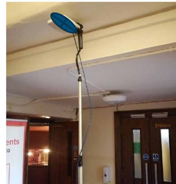
Location AP 36 - Upper Circle - unit installed at high level with other equipment and in close proximity to existing conduit.
