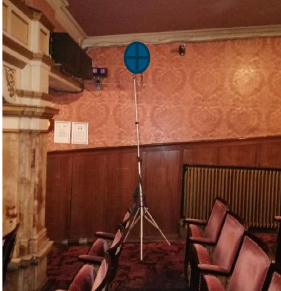
Location AP A4 - Stalls level - unit installed at high level close to existing cabling
