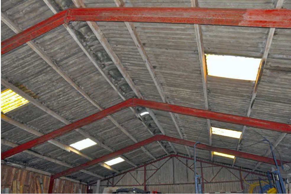
Internal view of main barn showing steel frame, open light conditions and lack of dark sheltered spaces suitable for use by roosting bats
