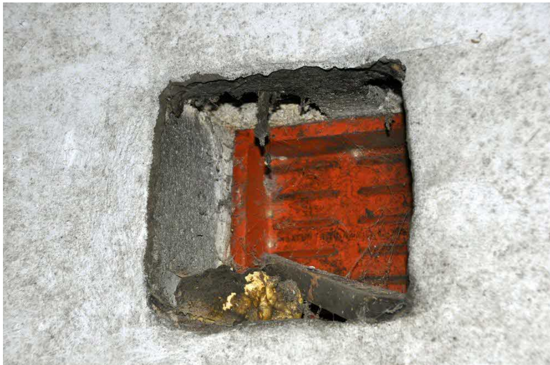
Old bird nest inside wall vent ledge inside stable block
