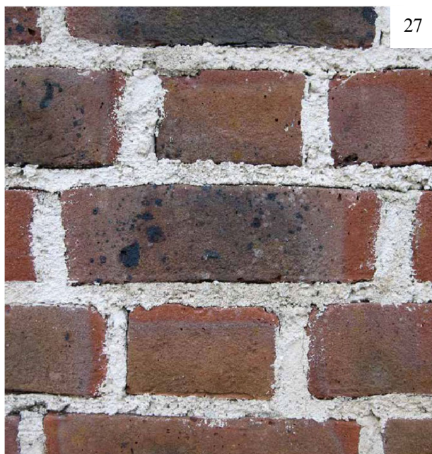
27. This shows a lime mortar which has been applied too wet. It has not been compacted and there is much shrinkage.
