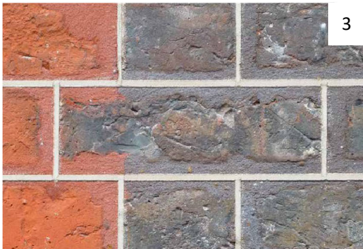
3. This shows an example of tuck pointing where wide mortar joints between unevenly shaped bricks are coloured to match the brickwork and a narrow 3-5mm joint of lime putty is then placed in scored grooves to create the impression of fine joints and uniform bricks.
