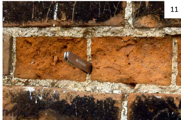
11. If a sharp tool can be driven into the surface of a lime mortar joint it does not mean that repointing is necessary. However, if there are open or poorly filled joints that offer no resistance at all then selective repointing will be required.
