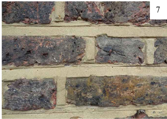
7. Weather-struck pointing to brickwork. This is slightly proud of the masonry and smoothed off at an angle.
