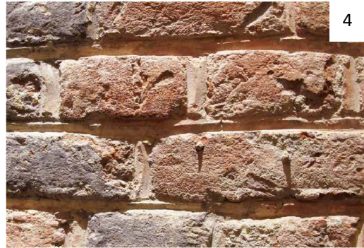
4. The mortar joint has been given a convex V-shaped profile which is referred to as beak or double struck pointing.
