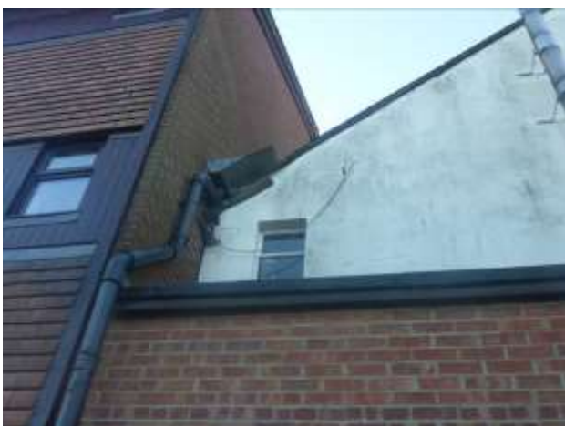
Photo 5: Gaps are present around lead flashing and where the building joins an off-site building.
