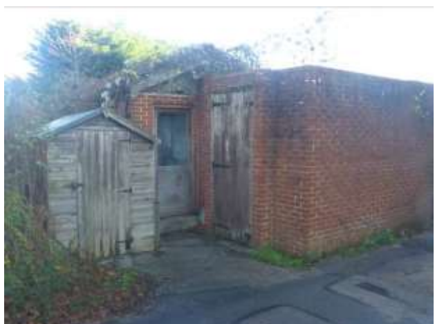
Photo 6: A collection of small outbuildings is present on the northern side of the site.
