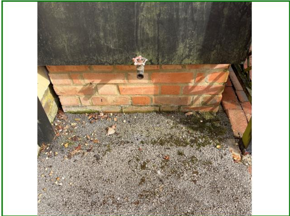
Photo No.16: Shows a close up of the tarmacked area under the oil tank.
