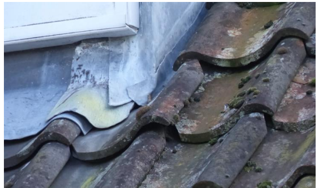
Close up of tile gap
