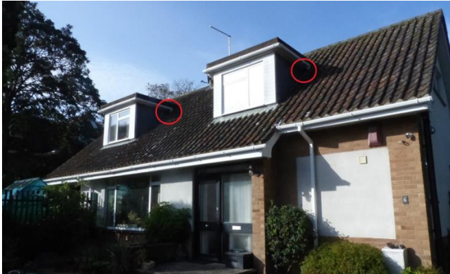
Location of gaps by dormers
