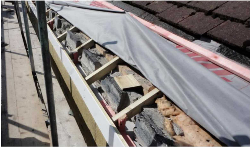
Figure 7 Roof eaves being extended example (Ref BRE External Wall Insulation (EWI) Report P107357-1000)
