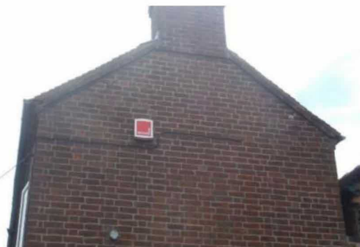
Figure 19 Gable end with insufficient overhang for EWI
