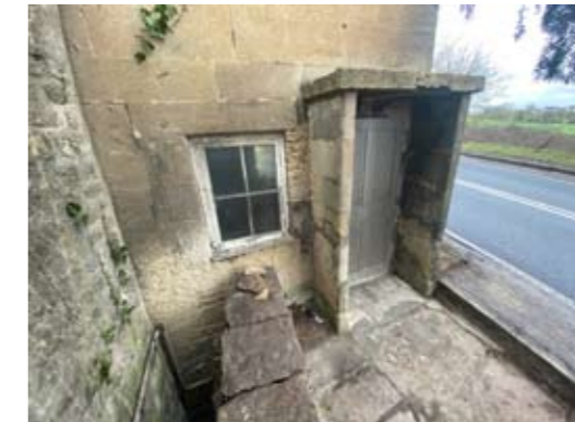
Left: Upper ground floor Toll House office View of the only original external door and window within the property
