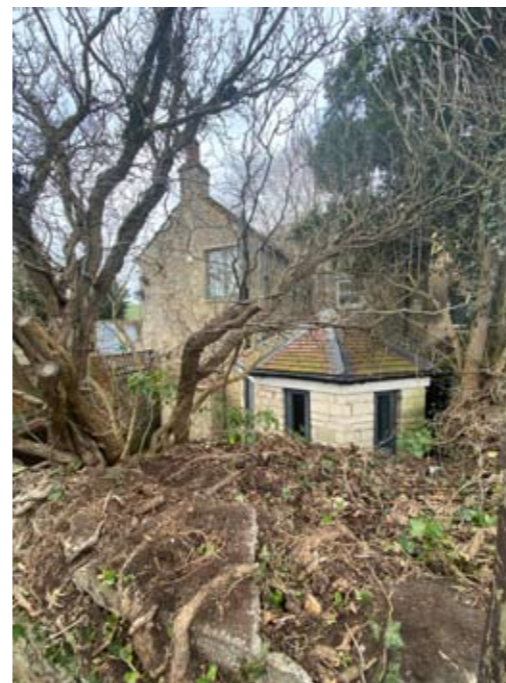
2006 Extension sits behind the old retaining walls, largely unseen from the road
