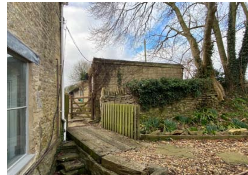
View of existing Annex - end North-east facade. The nearest of the Ash trees has since been removed - With Ash Die back
