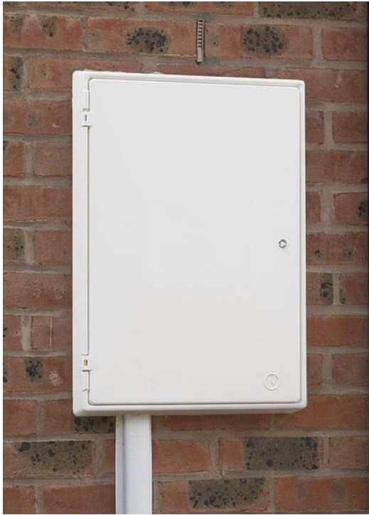
White flush electricity meter cupboard
