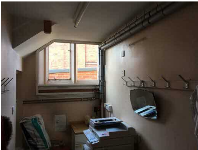
Existing office - wall to right to be removed to create larger kitchen.
