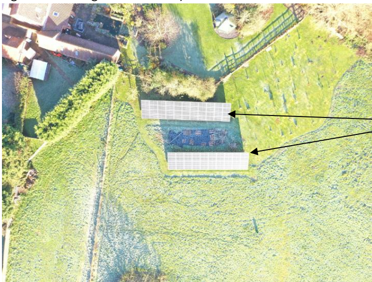
Figure 2: Existing solar PV array at site
