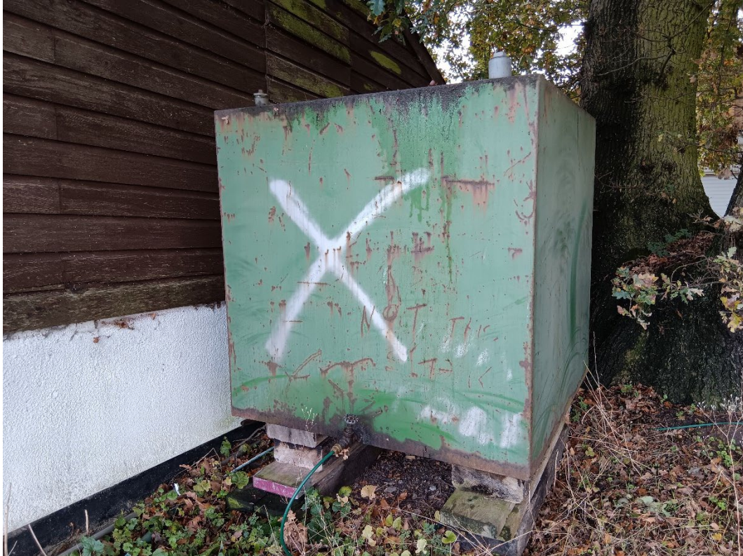
Off-site heating oil tank
