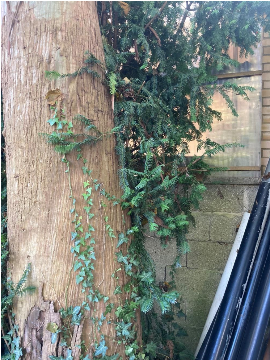
Photograph 3 Proximity of eucalyptus to party wall
