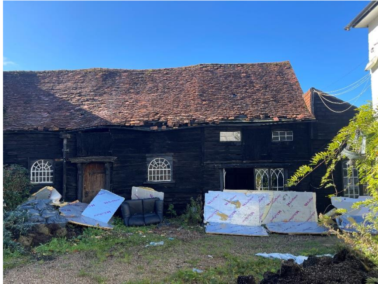
Fig 9. View of the barn with remnants of unauthorised use by third party
