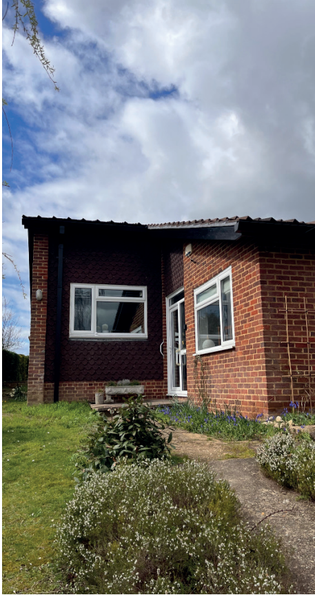
Tile Cladding to be replaced New aluminium window to replace existing PVC windows
