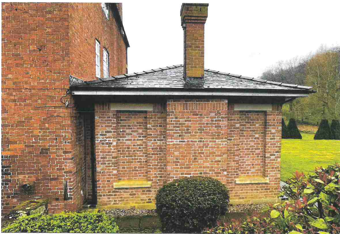
PHOTOGRAPH 13 - DETAIL OF THE DINING ROOM EXTENSION AS SEEN FROM THE REAR WHICH SHOWS THAT THE ROOF OVER THIS EXTENSION IS ALSO SHALLOW.
