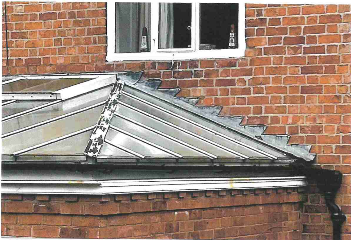
PHOTOGRAPH 7 - DETAIL OF EXISTING GLAZED ROOF WHICH SHOWS AREAS OF DECAY TO THE OUTER HIP.
