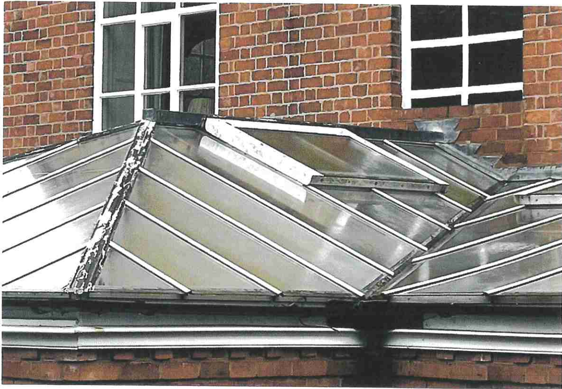
PHOTOGRAPH 6 - DETAIL OF EXISTING GLAZED ROOF WHICH SHOWS AREAS OF DECAY TO THE INNER HIP.
