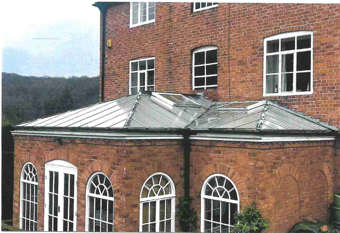
PHOTOGRAPH 3 - DETAIL OF THE EXISTING GLASS ROOF WITH ITS CONFIGURATION OF VALLEYS AND HIPS.
