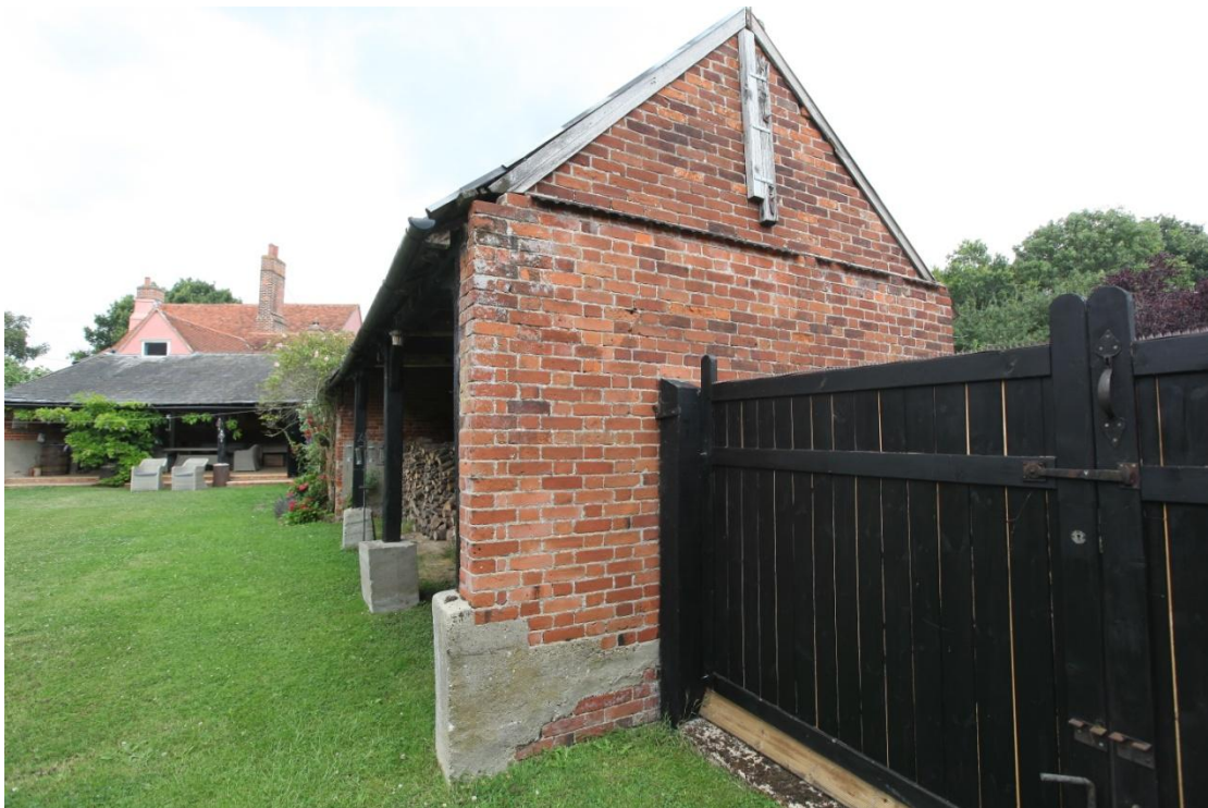
Illus. 12. The original Flemish Bond external southern gable of the horse yard's shelter-shed (1) at the southern end of the outbuilding.
