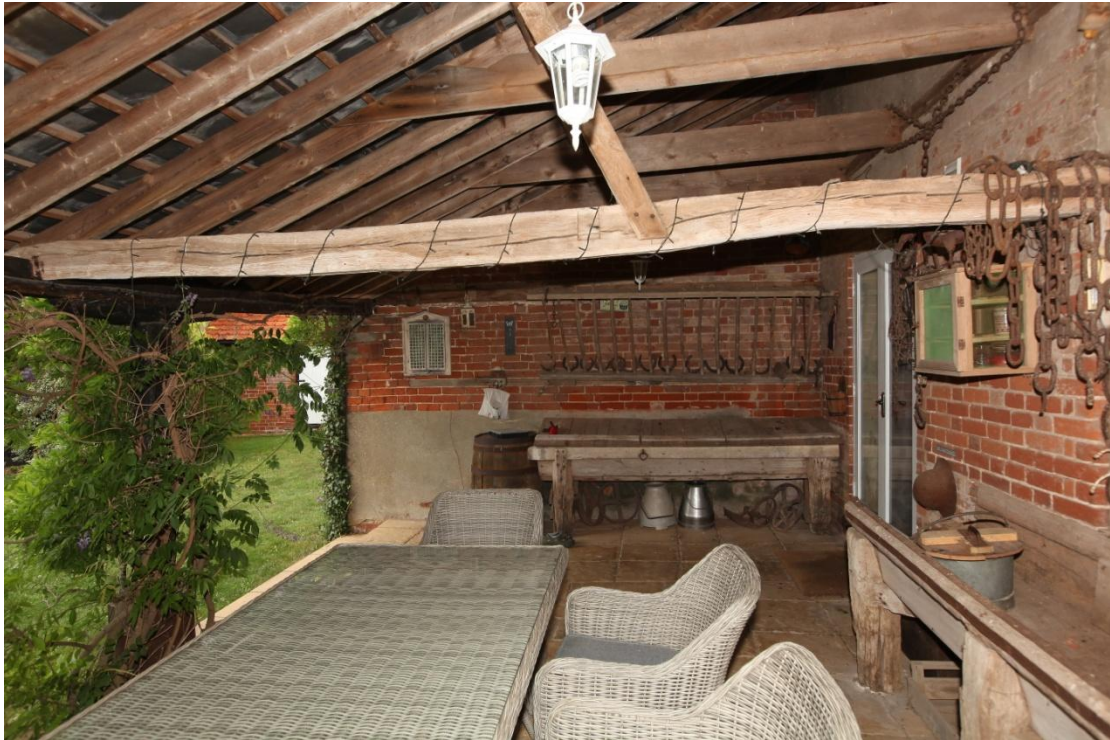
Illus. 35. The interior from the east of the shelter-shed to the cow yard (3) showing its open southern elevation on the left. The narrow-sectioned common rafters are 20 th century softwood replacements. This roof is a single-pitch structure adjoining the tall brick wall that divided the farm yard from the house on the right.
