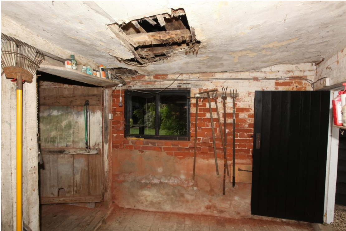
Illus. 29. The western interior of the mixing house (2a) showing the original plank-and-batten door to the main cow shed (2) on the left with the renewed door to the house on the right and the modern window to the shelter-shed (3) in the centre.
