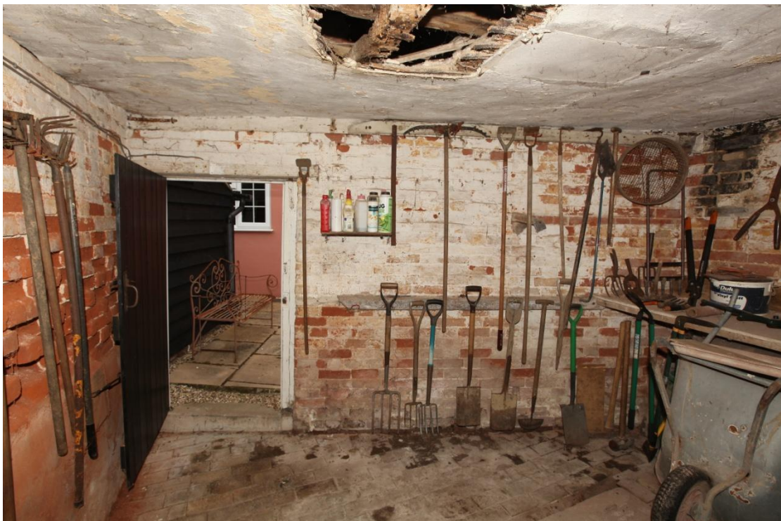
Illus. 28. The brick northern internal gable of the mixing house (2a) showing the original doorway which communicated with the house.
