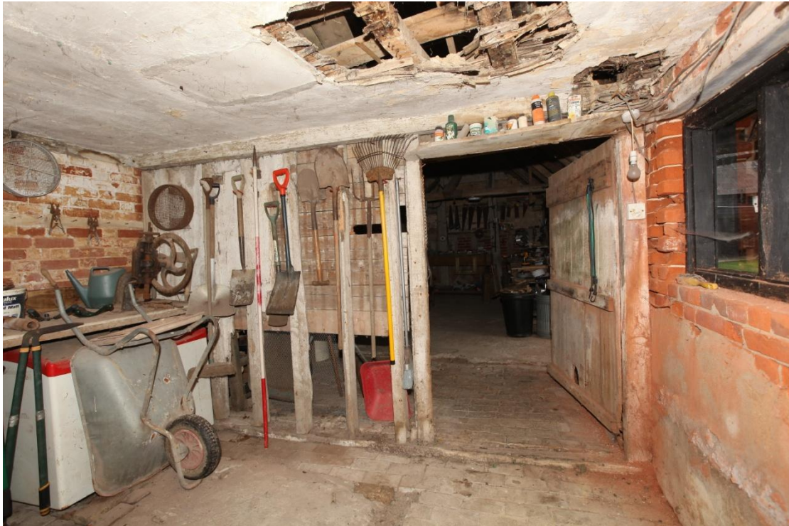
Illus. 27. The southern internal partition of the mixing house (2a) consisting of vertical studs with sections of original plaster surviving to the left. The exposed boards on the right retain the scars of nailed vertical laths to which the plaster was secured. Boarded walls were often sealed or ‘torched’ in this way in the 18 th and early-19 th centuries.
