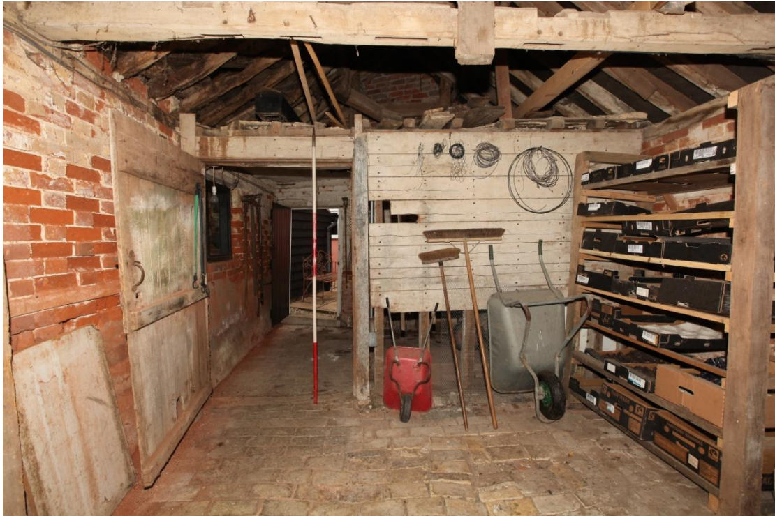
Illus. 21. The boarded partition and door of the mixing house (2a) at the northern end of the cow shed as seen from the south with the empty mortices of a re-used tie-beam in the foreground. The external gable door lies in the rear and the joist ends of the unusual double ceiling are visible at top right with details in illustrations 22-23.
