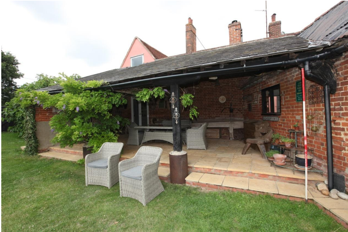
Illus. 31. The southern exterior of the three-bay open-fronted shelter-shed to the former cow yard (3) showing its slate roof and two intact arcade posts on later bases.
