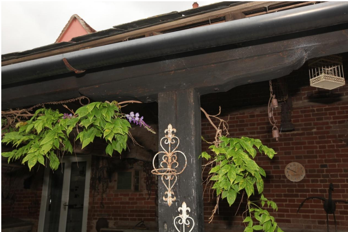
Illus. 32. A detail of the original shaped lintel dividing the arcade post of the cow-yard's shelter-shed (3) to the right in illustration 31 from its roof-plate.
