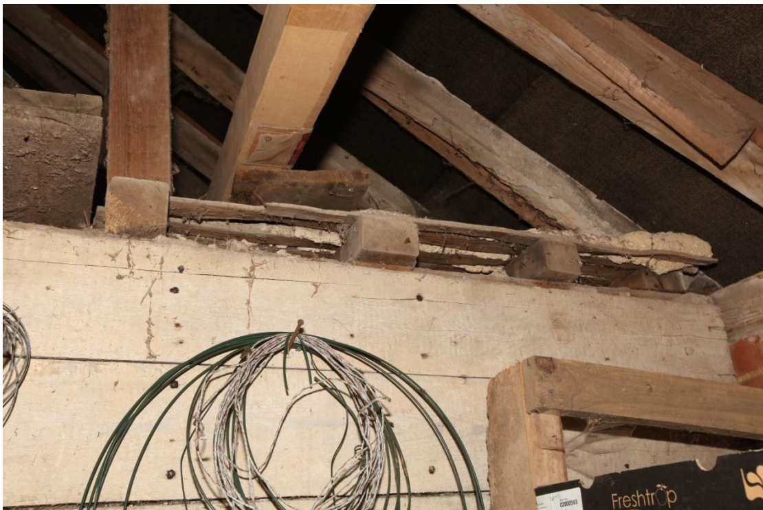
Illus. 22. A detail of the joist ends above the boarded southern wall of the mixing house in illustration 21 (2a). A small section of the original split laths of a daub attic 'floor' remains in situ . The attic floors of farmhouses were often constructed in this way when there was no access to the attic rooms and therefore no need for floorboards. They offered additional protection from dust and water ingress from above.
