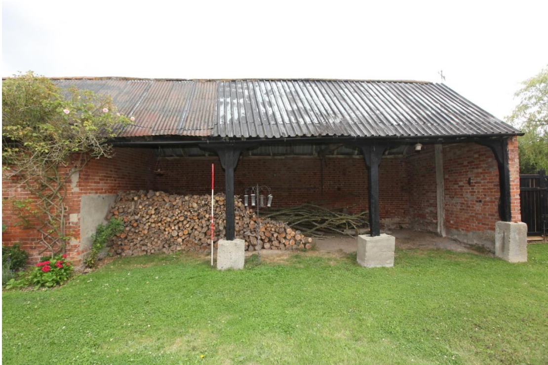
Illus. 13. The open western wall of the three-bay shelter-shed (1) that formerly served the horse yard adjoining the stable (as described in 1938 and shown on the Ordnance Surveys). The two original wooden arcade posts survive along with all four knee-braces, but their feet have been encased in concrete blocks. The roof consists of a mixture of corrugated iron and modern pressed metal.
