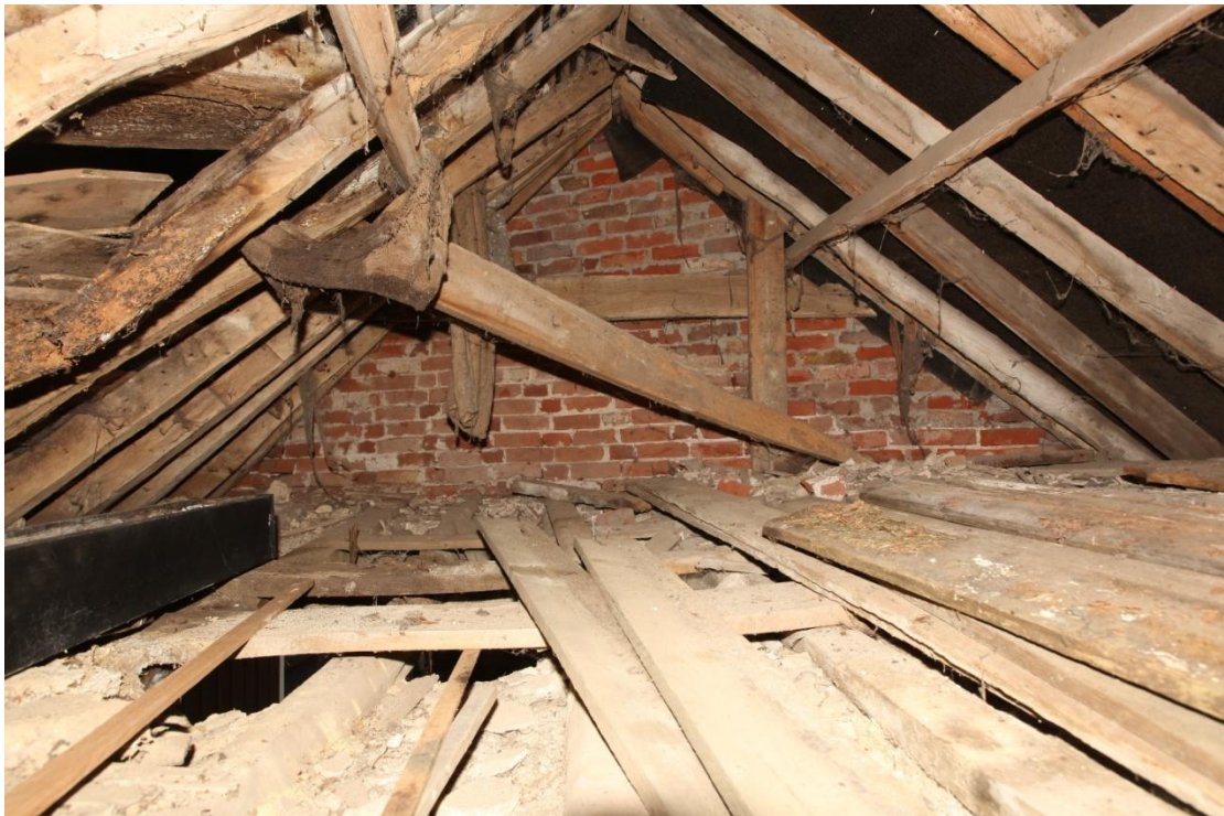
Illus. 24. The roof space above the mixing house (2a) at the northern end of the cow shed showing its gable in the rear. Most of the original clay daub floor in illustration 23 has been lost and boards have been laid across the joists instead. This space appears to have been accessible from the cow house (2) and may have served as a hay or straw loft. The clay floor prevented its contents from damaging the lath-and-plaster beneath.
