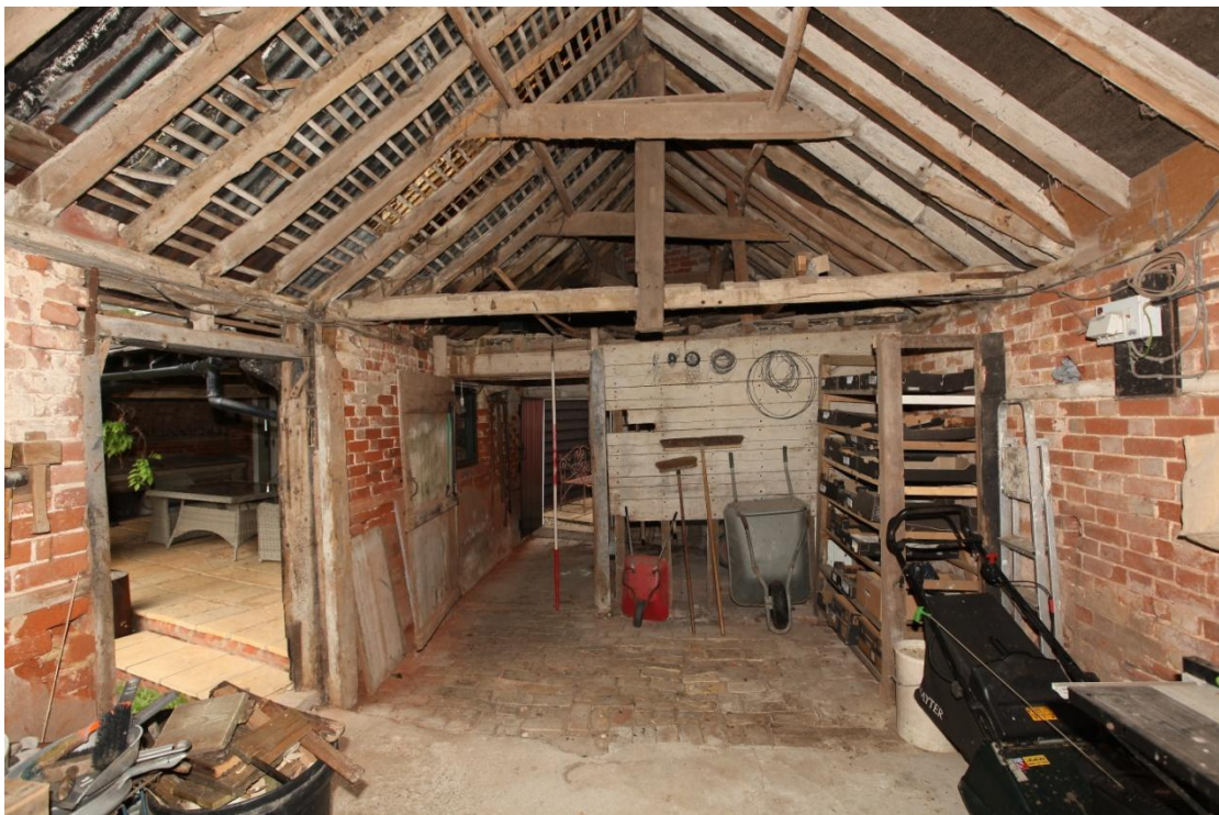
Illus. 20. The interior from the south of the cow shed (2) showing its original wide doorway to the missing enclosed cow yard on the left. The boarded partition of the feed mixing house (2a) is visible in the rear along with a section of original floor bricks.
