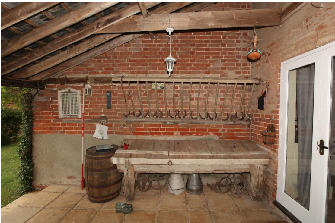
Illus. 36. The western interior of the shelter-shed that served the cow yard (3) showing a 19 th century hay rack with wooden tines above a low boarded manger of the same period. The French doors on the right are 20 th century insertions that connect the building directly to the house.
