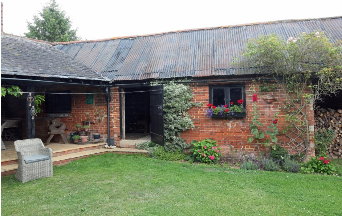
Illus. 17. The western exterior of the brick cow shed (2) showing its wide entrance door on the left. Both the door and window apertures are respected by closers (quarter-bricks) and are original to the wall fabric – although the window and door are modern replacements.
