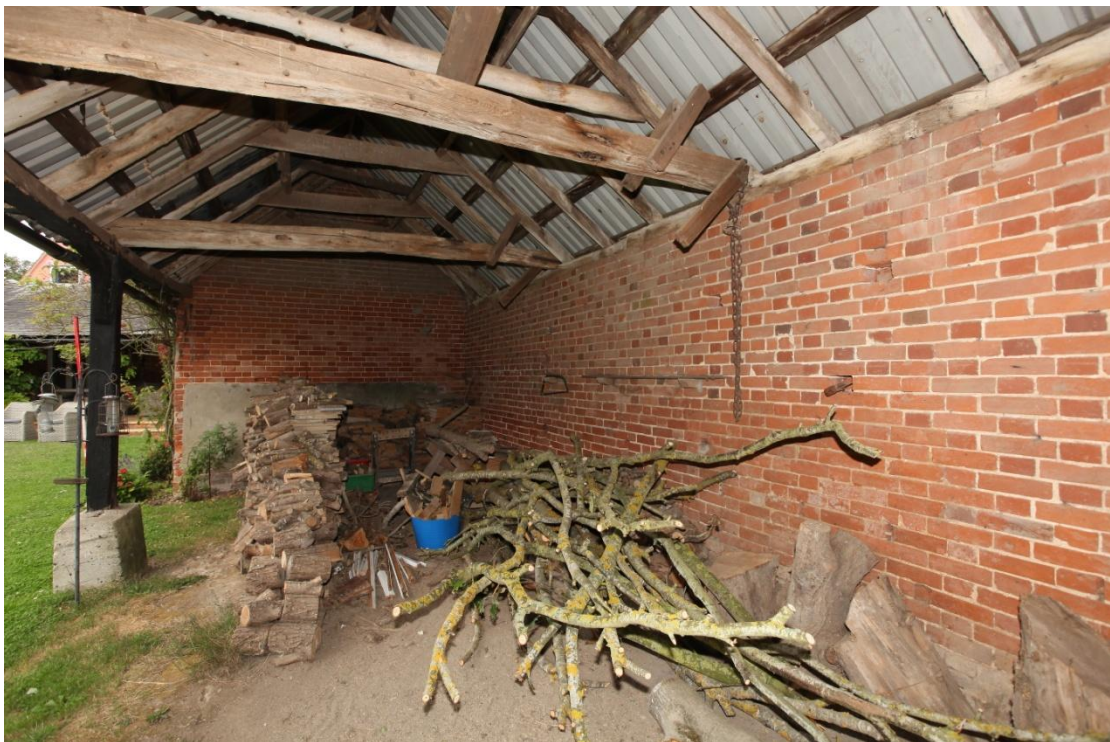
Illus. 14. The interior of the horse shelter-shed (1) from the south showing the re-used timber of its tie-beam that may have been salvaged from the earlier farm buildings on the site. The wooden troughs in the cow shelter-shed (1) are understood to have been removed from this space.
