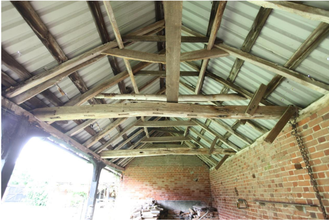
Illus. 15. The roof structure of the horse shelter-shed (1) from the south showing the empty pegged mortices of the 16 th or early-17 th century re-used tie-beam in the foreground. The original roof collars are nailed rather than pegged and the majority of the rafters have been removed.
