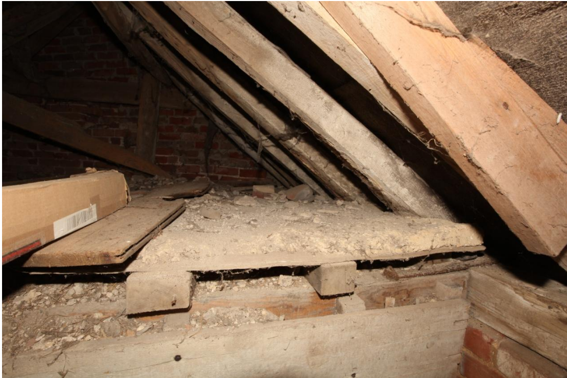
Illus. 23. A further detail of the rare original 'floor' of clay daub to the roof void above the mixing house (2a), consisting of a thick layer of clay, straw and hair applied to split oak laths laid across the joists. The lath-and-plaster of the inner ceiling is also visible beneath the joists.
