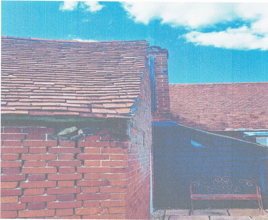
P5 –Crack to flank wall and leaning (outward) north gable wall to storeroom.
