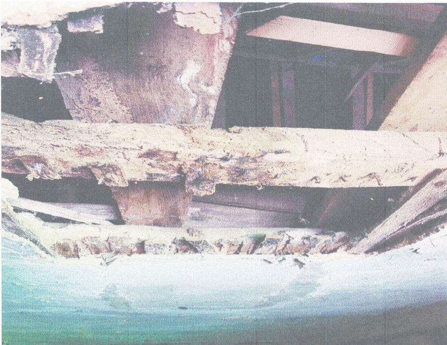
P8 – Decay to timber ceiling joist over storeroom.
