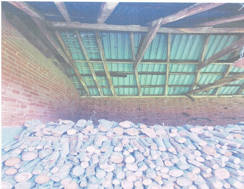
P4 – Skewed rafters to cart lodge due to racking and leaning gable wall of workshop.
