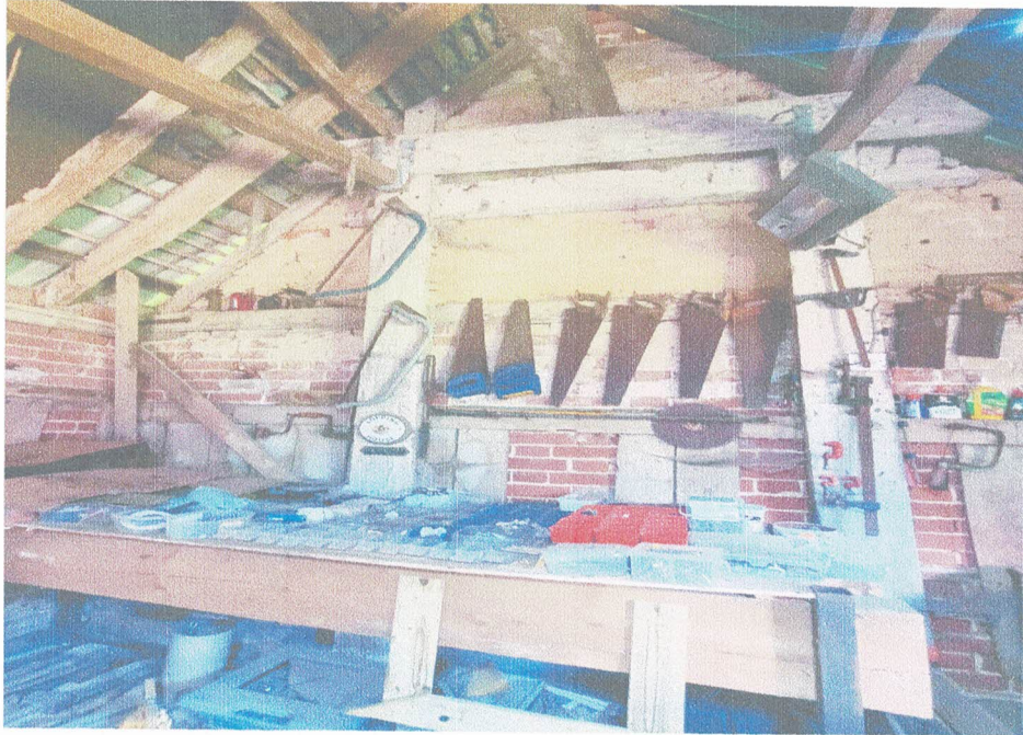
P3 – Propping to leaning (inward) south gable between workshop and cart lodge.
