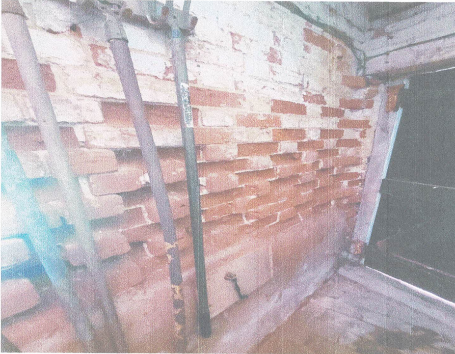
P7- Brick loss storeroom wall adjoining covered patio area.
