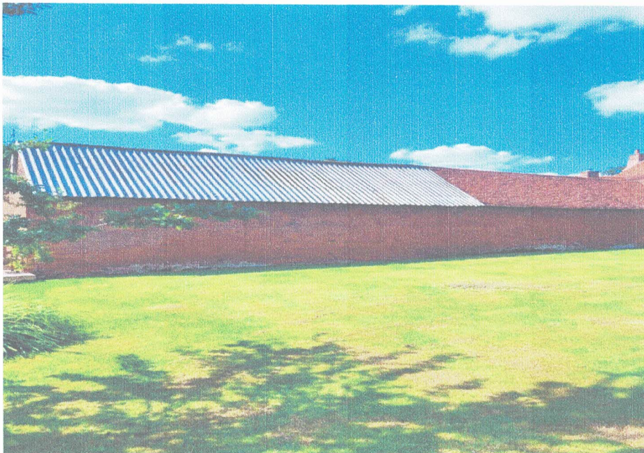
P2 – General view of rear elevation of cart lodge (corrugated roof ) and workshop (tiled roof).
