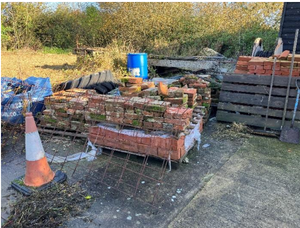
Photo 11: Building materials stored on raised pallets
