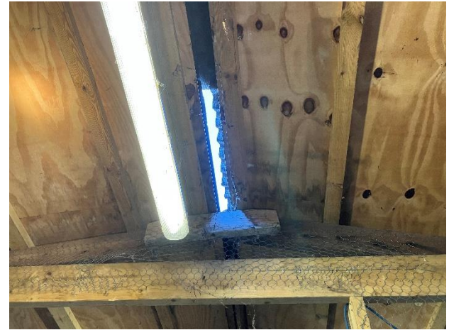
Photo 6: Missing ridge covering on main building section
