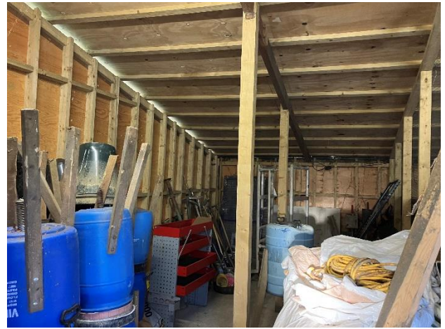
Photo 4: Internal view of main building – a modern wooden frame covered with plyboard and weatherboarding
