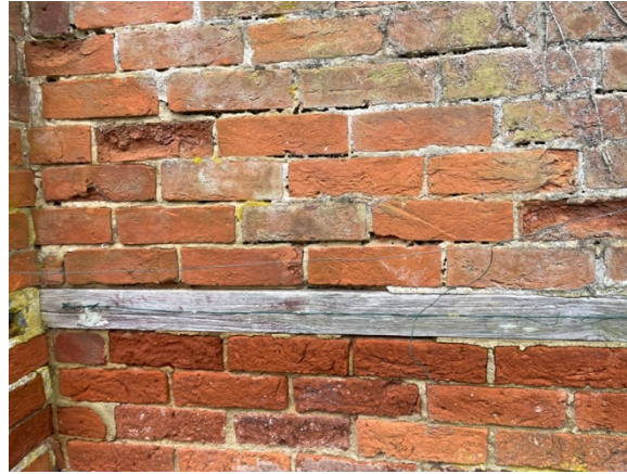
Photos showing the poor condition of the existing pointing to the rear outbuilding.
