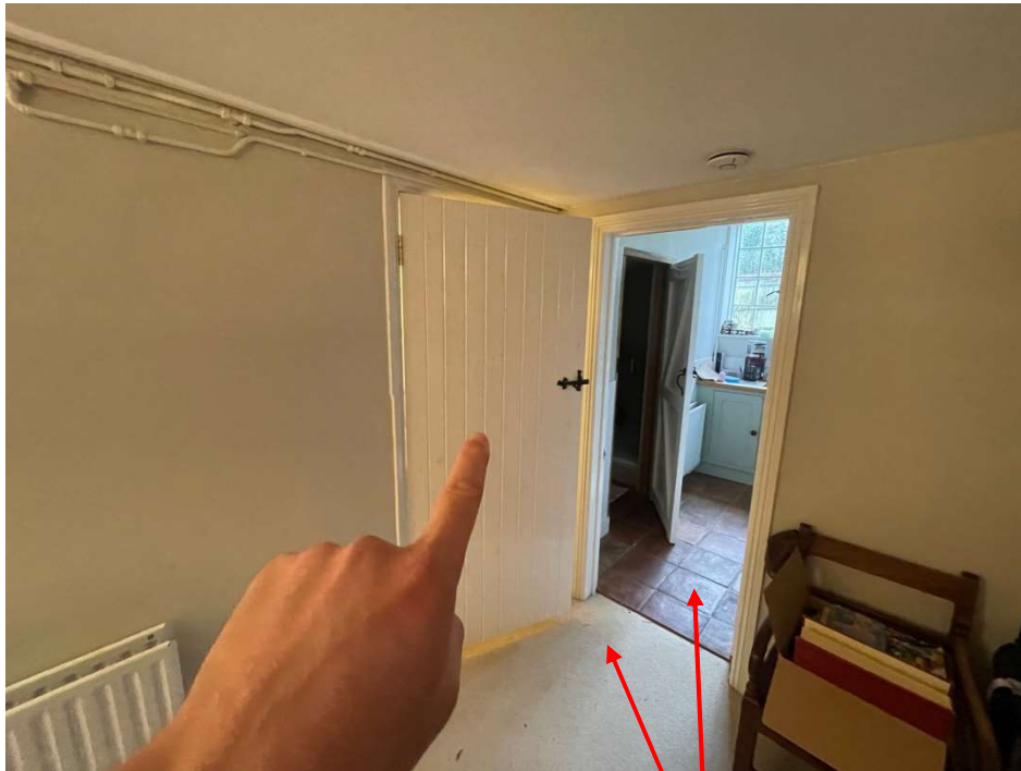
Existing door to be removed. Doorway to remain and reveal made good
