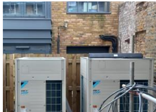
Fig3. View from ground floor level flat when opening windows and leaning out on window sill (Please note this picture was taken during construction works)
