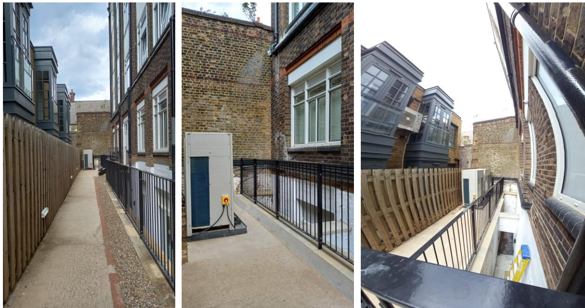
Fig1. Existing view of the installed ac units, including from the rear access/egress of core A
