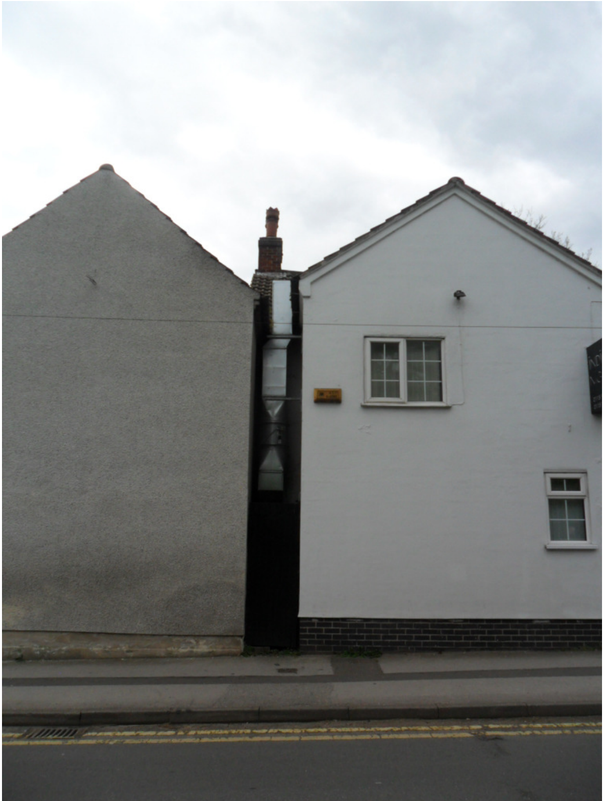
EXTRACT DUCTING TO BE REMOVED; adjacent gable since demolished; will be replaced by new development
