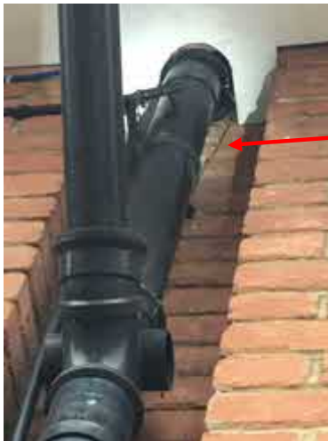
Photograph 25. Gap around downpipe with vegetation
