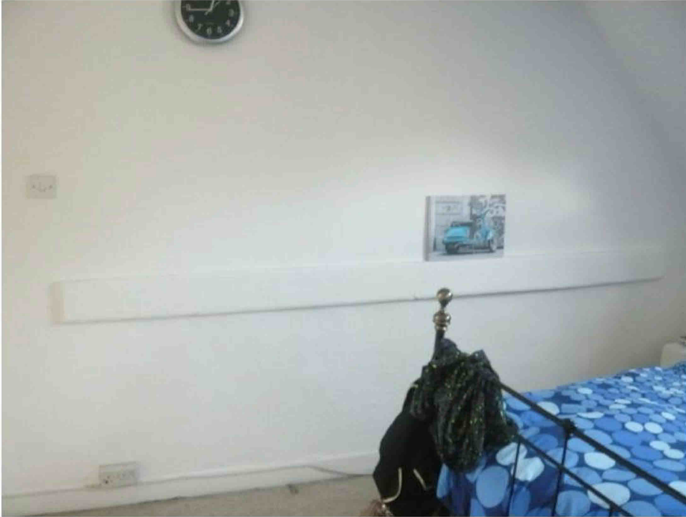
Fig.12 Truncated tie-beam within the north wall of the southernmost room in the front range
