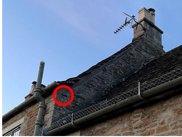
Photo 2 – Building 2, A rot hole where common pipistrelle and brown long eared were recorded emerging and re-entering
