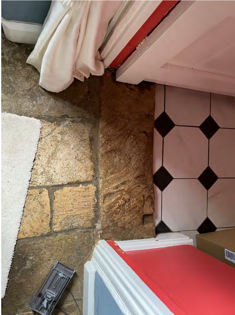
Plate 19: Worn stone threshold and level change between GF7 and GF8.
