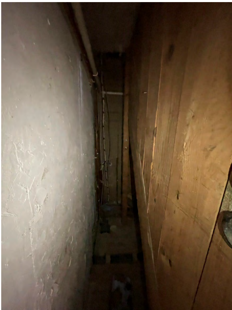
Plate 28: Void on the south side of the staircase between the first and second floor (FF9).
