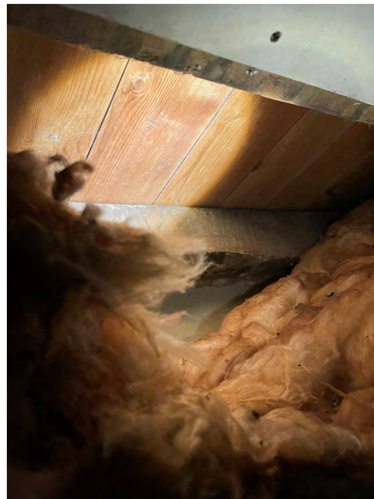
Plate 25: Detail of modern pine floor boards of GF2 as seen from the cellar below.
