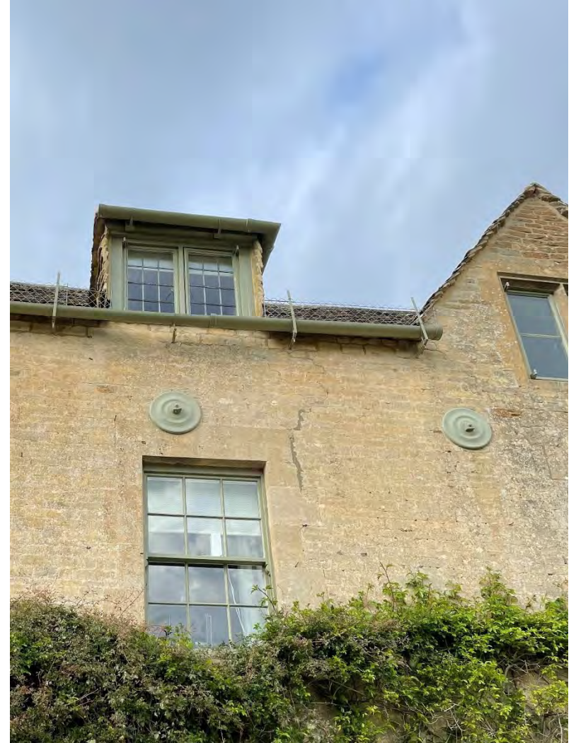
Plate 21: Detail of first floor and roof level of the south elevation of the central bays.
