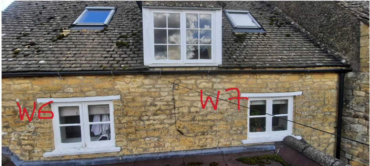
EXISTING REAR ELEVATION – VIEWED FROM STANDING ON FLAT ROOF, SHOWING WINDOW NUMBERS
