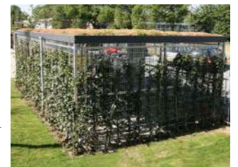
Example of a bin store with a green roof and mesh cladding panels with climbers growing on them. Good for visibility.
