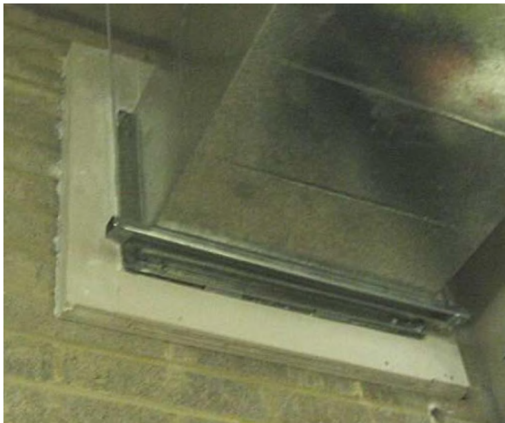
Figure L-5 - Duct penetration with gypsum cover plate site photo
