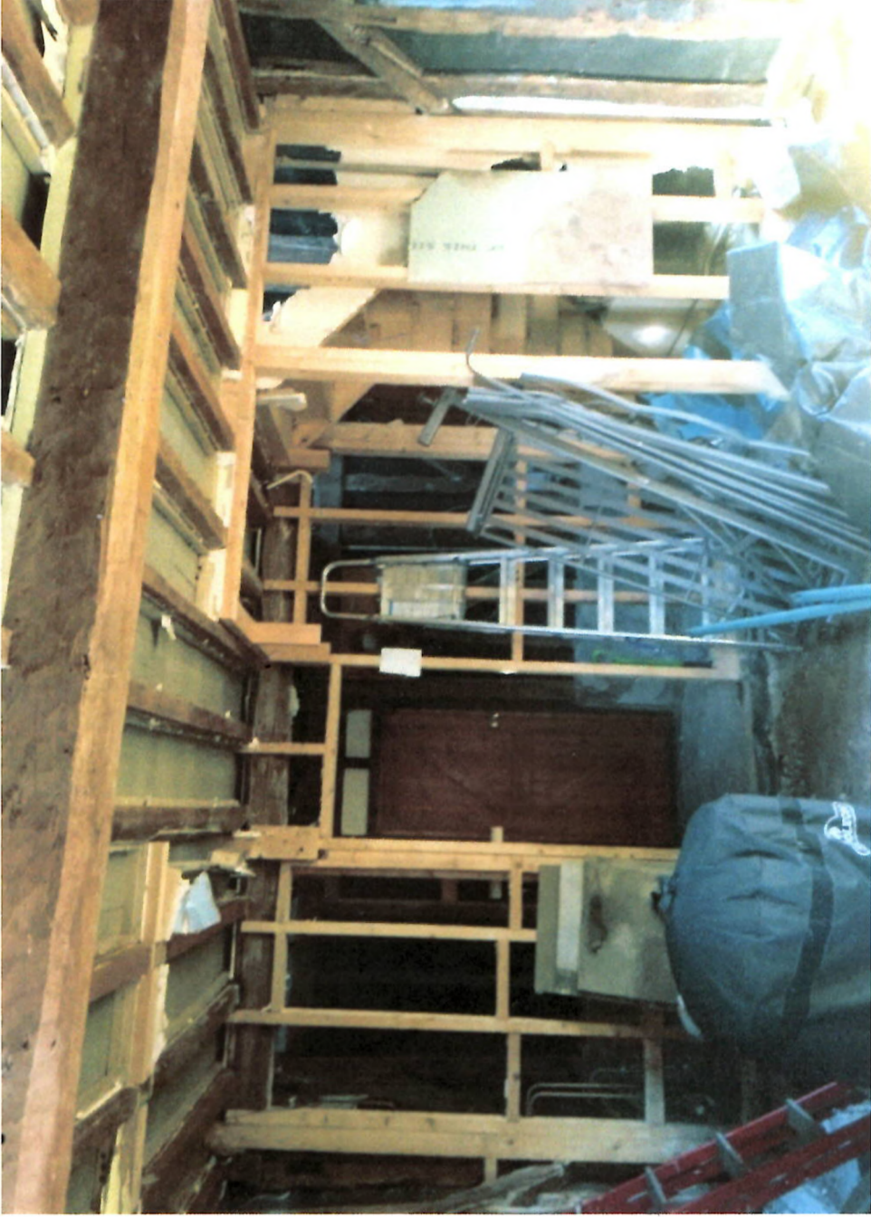
INTERNAL GROUND FLOOR VIEW WESTWARDS SHOWING THE ABANDONED BUILDING WORK TO THE EXISTING BARN DWELLING (TO BE CONVERTED).
