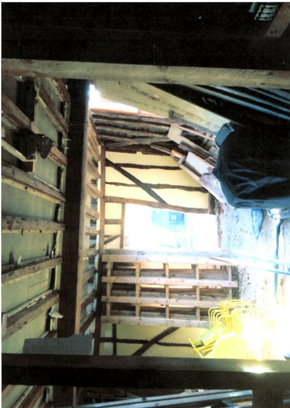
INTERNAL GROUND FLOOR VIEW EASTWARDS SHOWING THE ABANDONED BUILDING WORK TO THE EXISTING BARN DWELLING (TO BE CONVERTED).
