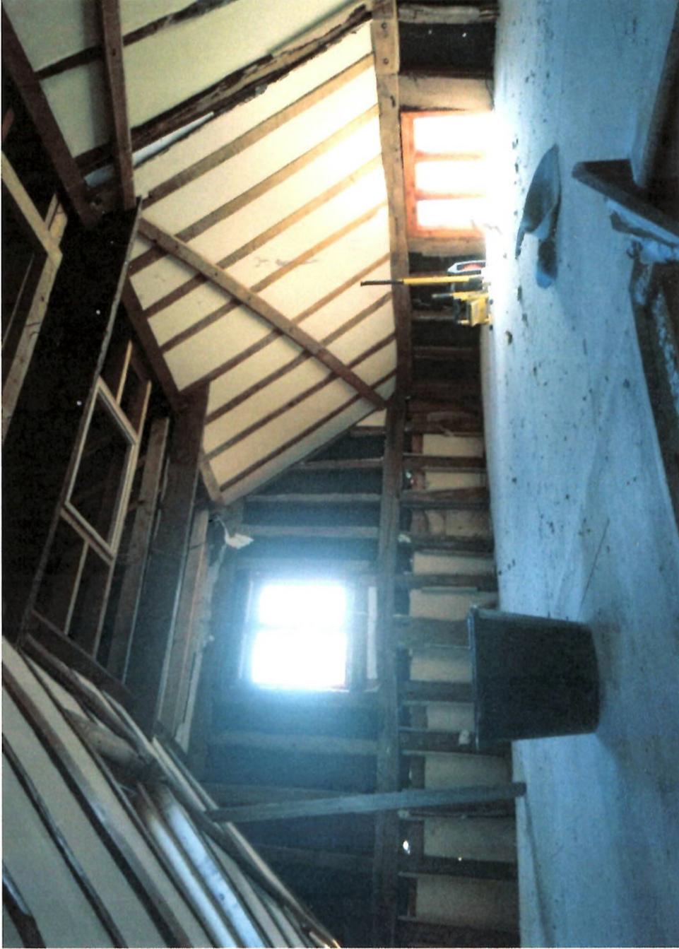
INTERNAL FIRST FLOOR VIEW EASTWARDS SHOWING THE ABANDONED BUILDING WORK TO THE EXISTING BARN DWELLING (TO BE CONVERTED).
