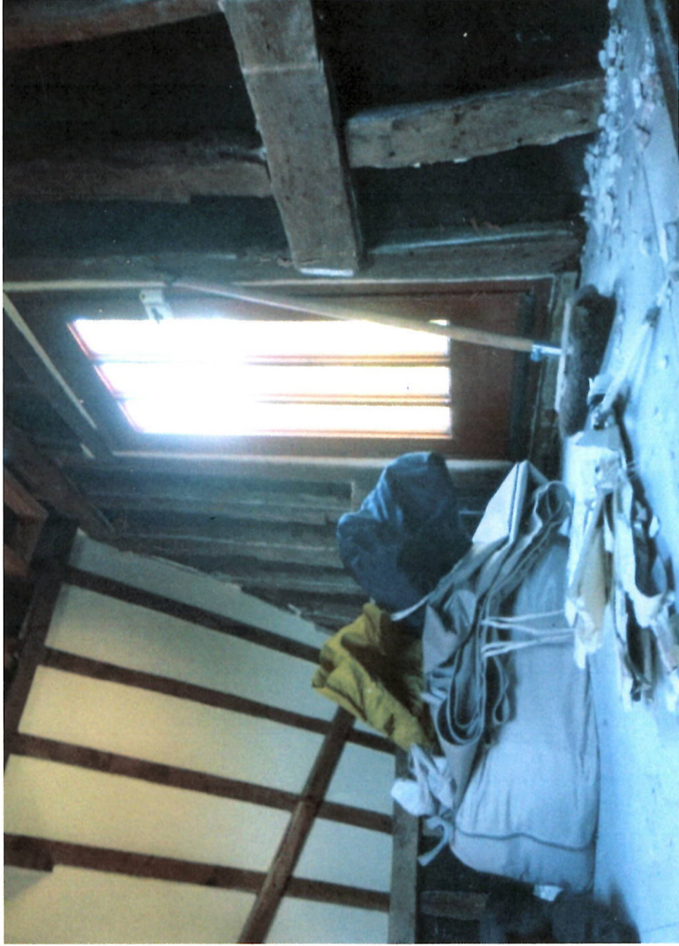
INTERNAL FIRST FLOOR VIEW SOUTH WESTWARDS SHOWING THE ABANDONED BUILDING WORK TO THE EXISTING BARN DWELLING (TO BE CONVERTED).
