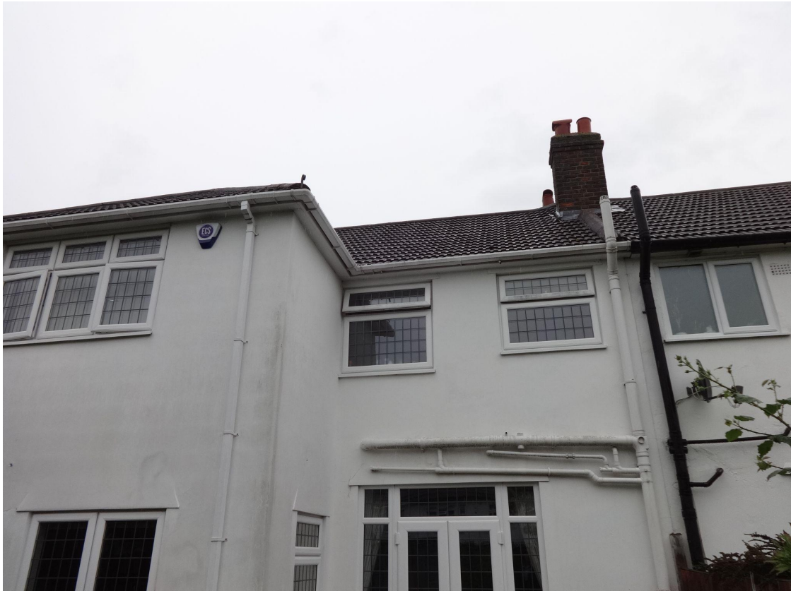
Fig.2 Existing rear elevation with number 65 Gloucester Avenue indicating bathroom window referenced above
