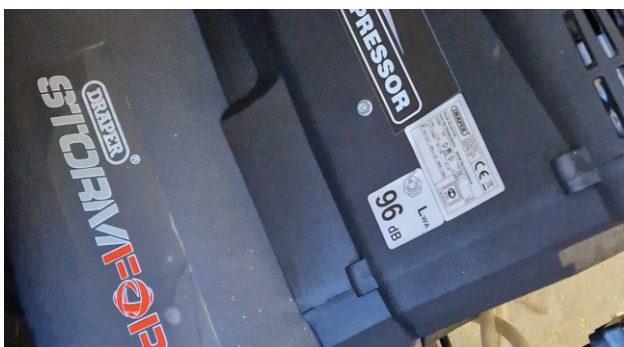
Existing air compressor within unit 15
