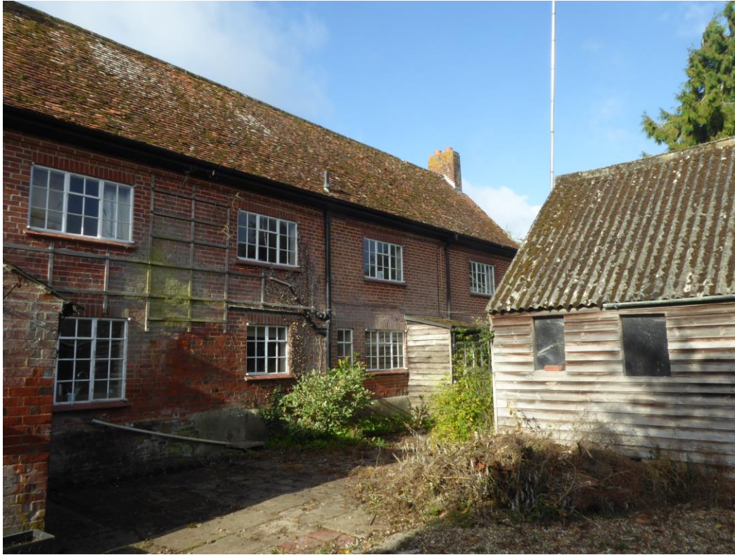
Fig 9 – View of the rear elevation of the house and the C20 one storey extension.
