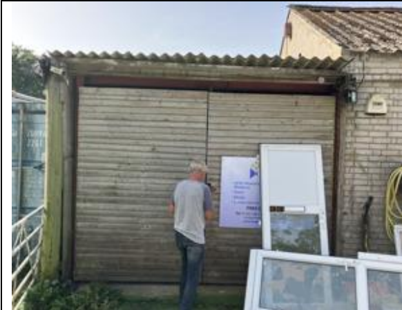
Photograph 11. The store on the rear of the garage and workshop with a large gap at the top but tight weatherboarding.
