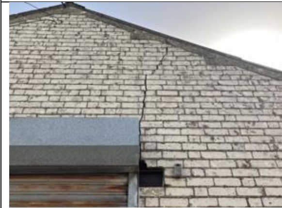
Photograph 17. A large crack with potential to support crevice dwelling bats
