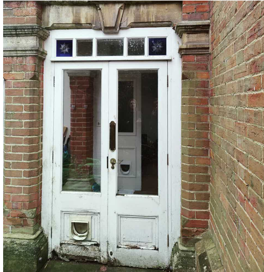
Figure 13. View of damage to the double doors on the North elevation.
