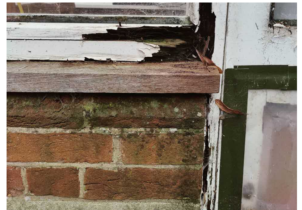
Figure 16. Damage at the junction between the glazed link door and the plinth.
