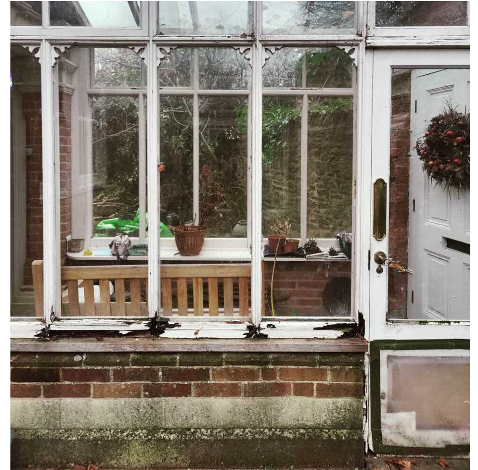
Figure 14. View of damage to the glazed link from the courtyard.
