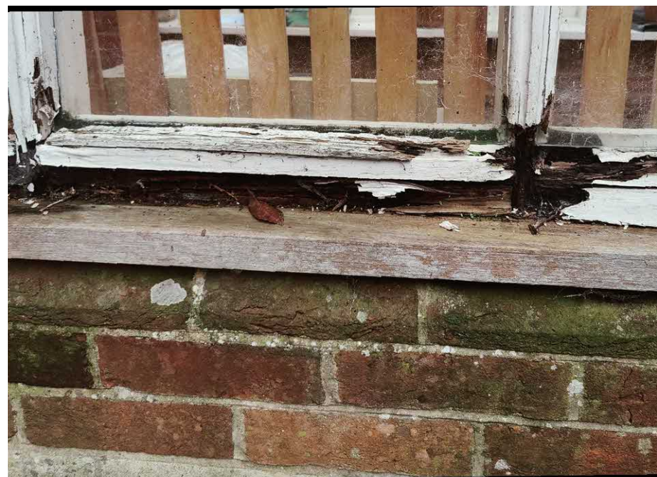
Figure 15. Damage at the junction between the glazed link and the plinth.
