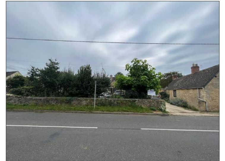
EXISTING WALL IN DILAPIDATED STATE (ADJACENT SANTOY SEEN TO THE RIGHT)
