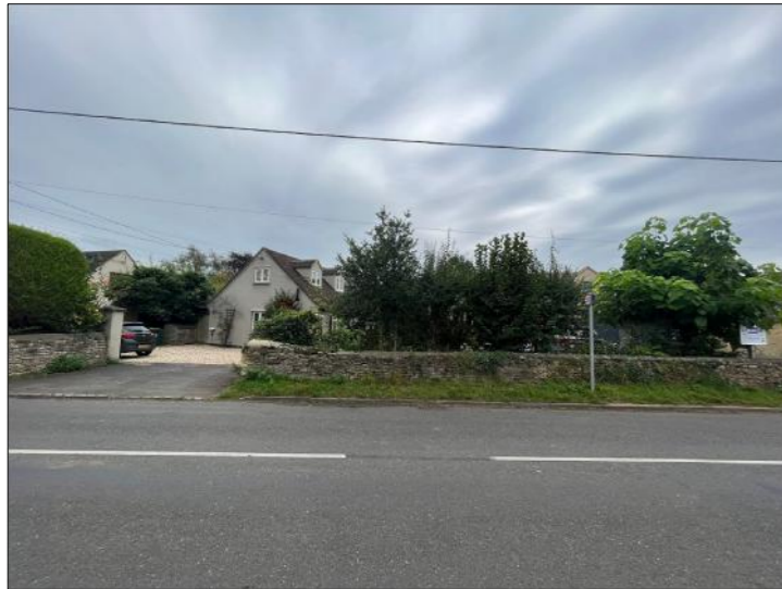
EXISTING WALL IN DILAPIDATED STATE (ADJACENT ROSEBROOK SEEN TO THE LEFT)
