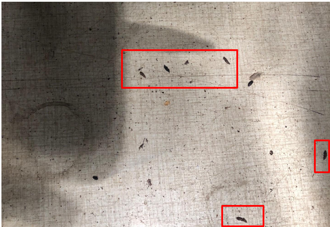
Photo 8 , bat droppings located within loft space.
