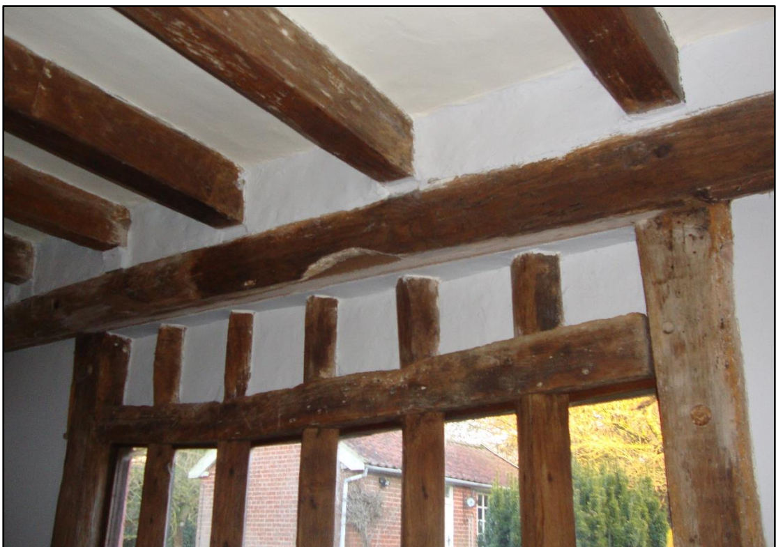
Fig.25 Mullions and central rail of original hall window with later inserted floor
