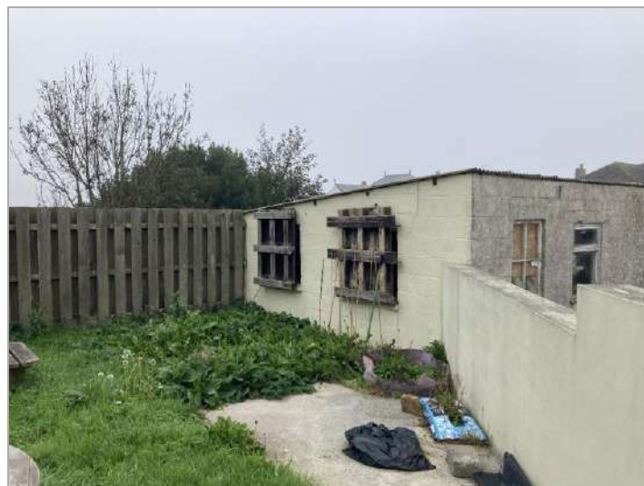
PHOTOGRAPH 6: View of a concrete block with corrugated metal roof outbuilding located in the north-western corner of the site
