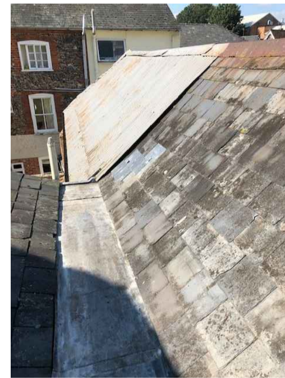
1. South slope: view of valley gutter and partial slate/partial steel roof coverings.
