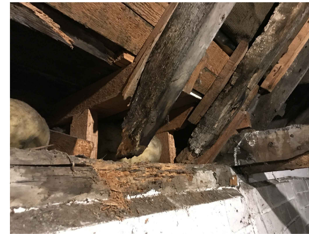
2. South slope: rotten rafters stop short of wall plate.
