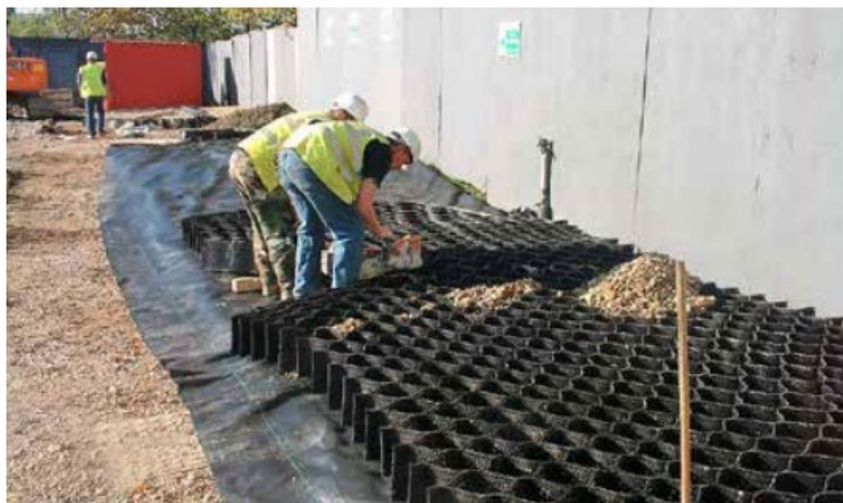
SGN 3-06 Cellular products are a very effective means of providing ground protection where heavy vehicle use is expected. Here, it is being used to temporarily widen an existing road, to be removed once the construction is finished.
