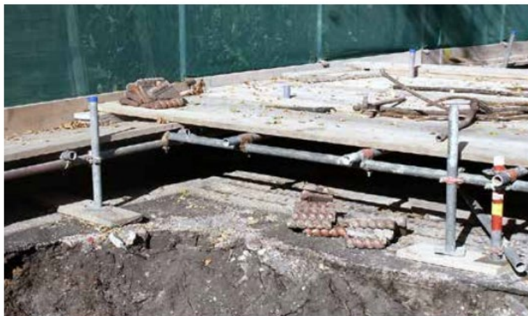
SGN 3-05 A scaffold framework attached to the main scaffold fencing can be used to support either scaffold planks or plywood to create an elevated platform with a gap beneath.
