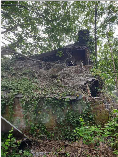
Photograph 3: Collapsed roof viewed from the west.
