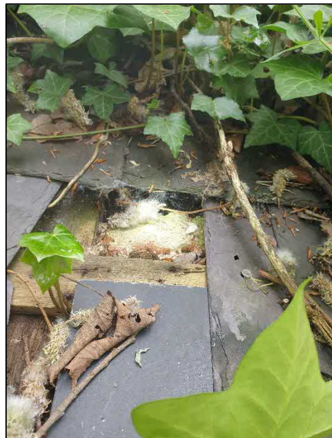
Photograph 4: Damaged roof slates with encroaching ivy.
