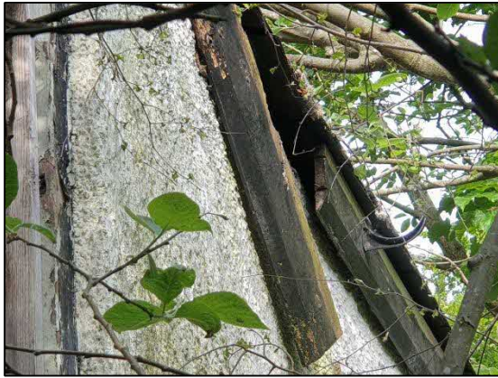
Photograph 5: Damaged fascia boards.
