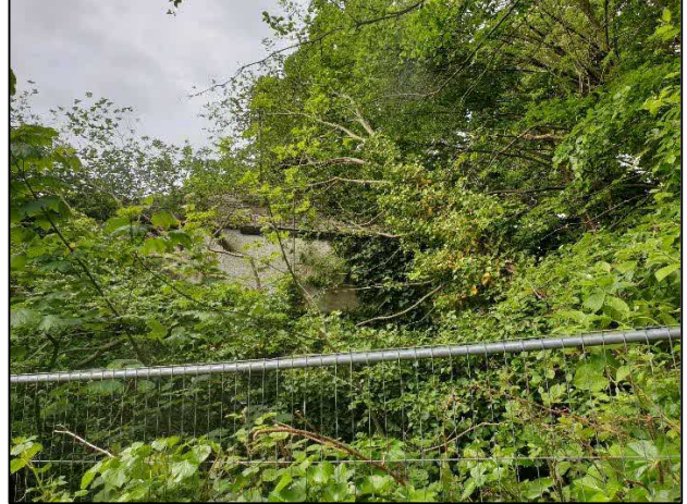
Photograph 2: The fallen tree and northern aspect of the building.
