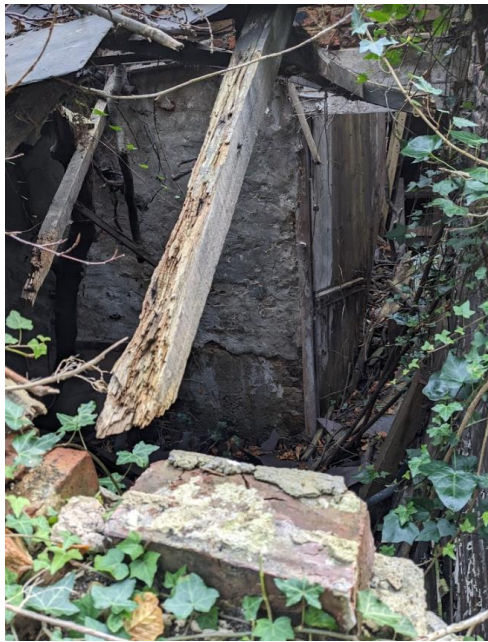
Figure 5 - Example of a rotten timber roof joist
