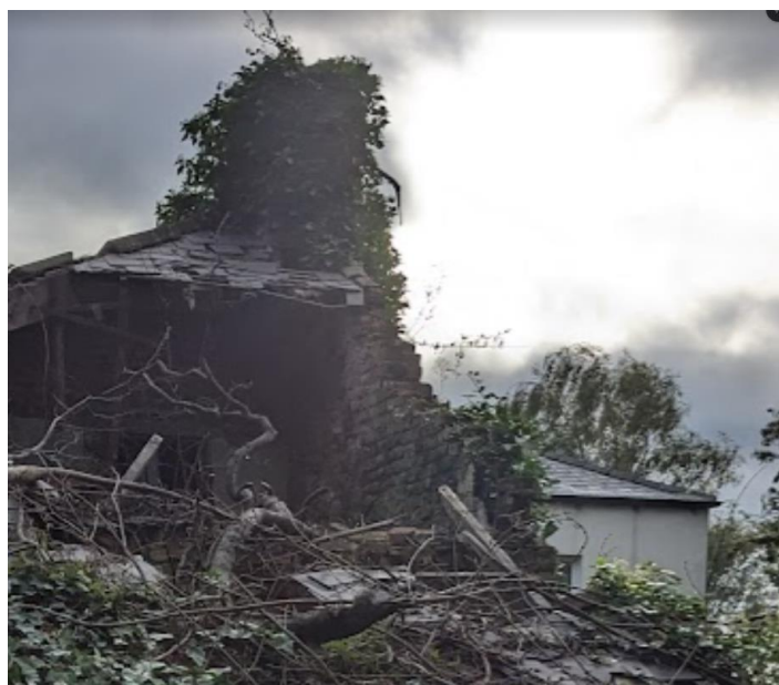
Figure 13 - Damaged section of south elevation
