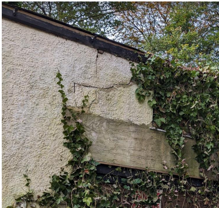
Figure 10 - Cracking over doorway on north elevation
