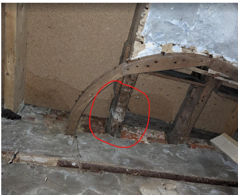
Figure 8 - Apparently rotten first floor joist
