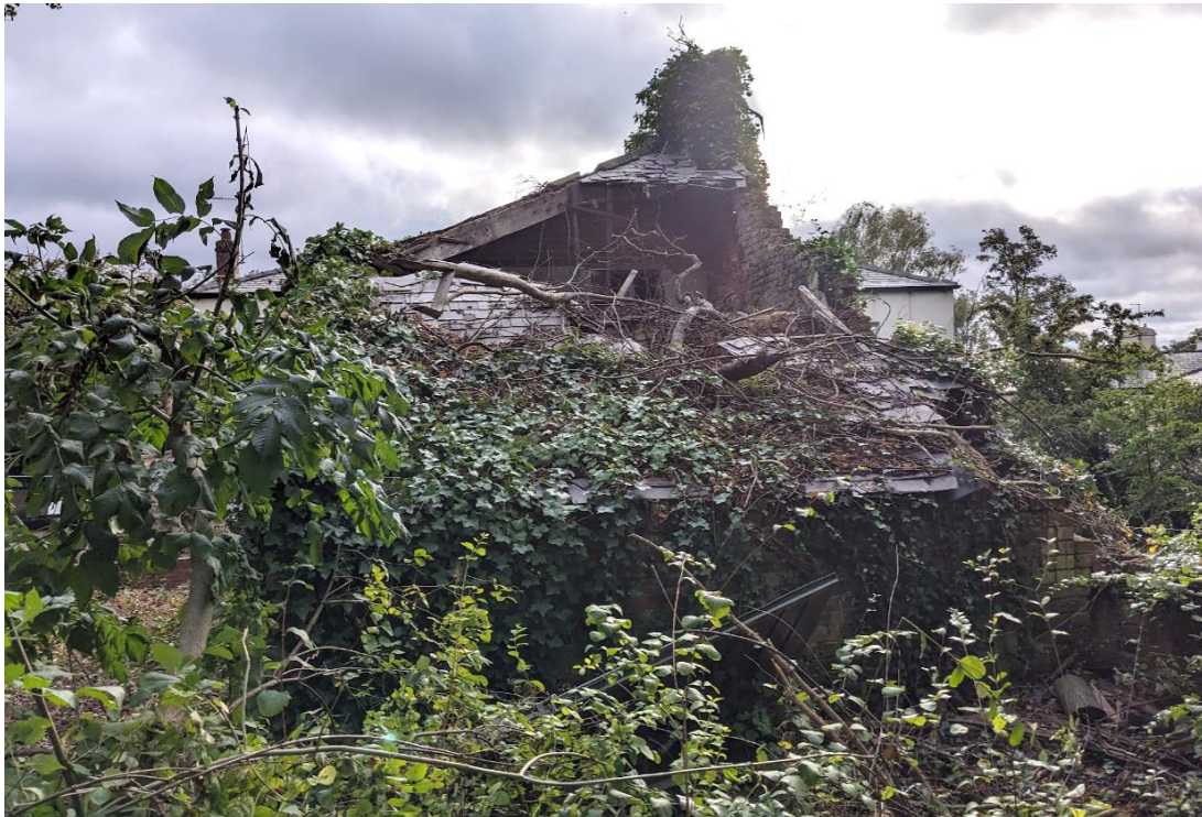
Figure 4 – View from the west of the collapsed section of roof
