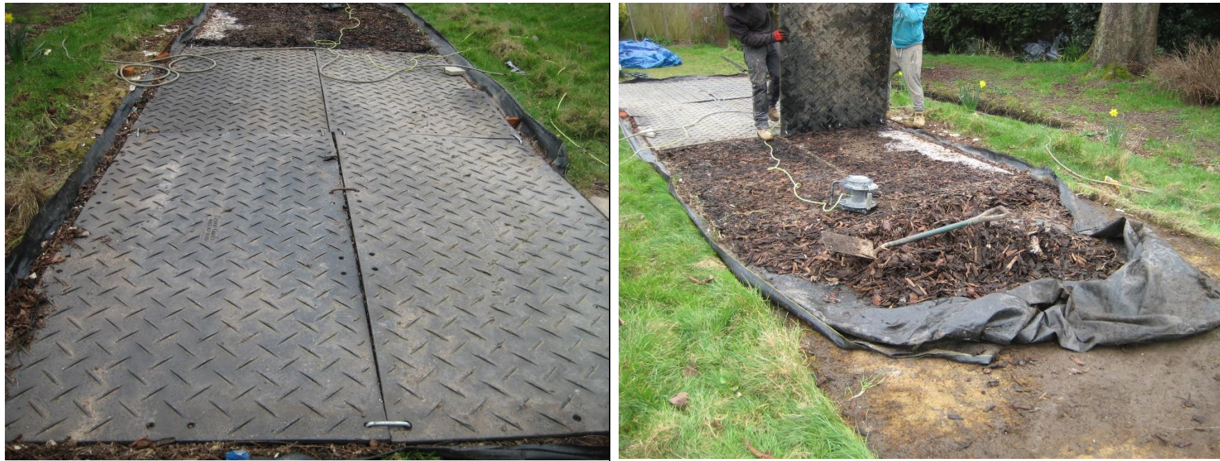
Fig 12 – Temporary ground protection is an effective way of allowing access through the RPA of retained trees. It must be installed prior to any on site activity and maintained for the duration of all works to be effective. Above left Tamla Trees project ground protection in place and above right being removed following the completion of site works. (Note: depending on the length of time it is in place it will adversely affect underlying grass ground cover which will need reseeded/ turfed accordingly)
