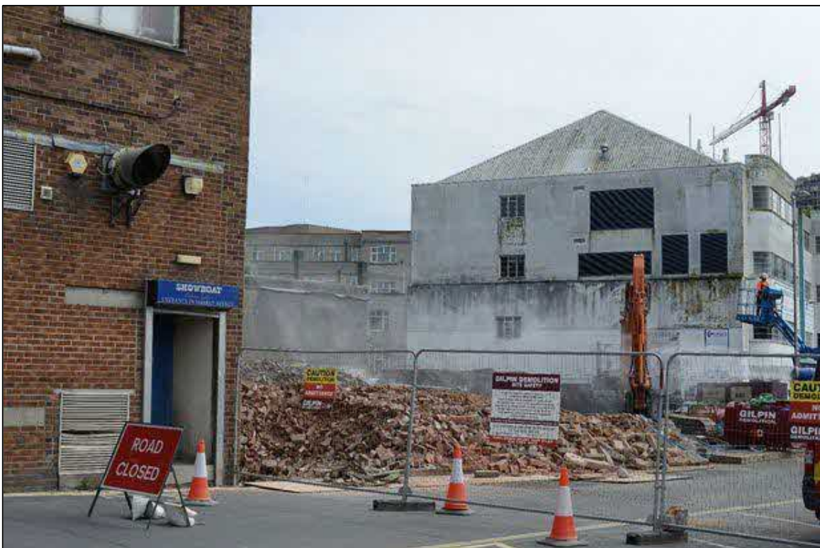
FIGURE 17: THE 2017 DEMOLITION WORKS WHICH REVEALED PREVIOUSLY OBSCURED WINDOWS ON THE SIDE ELEVATION; PLYMOUTH.LIVE.CO.UK.
